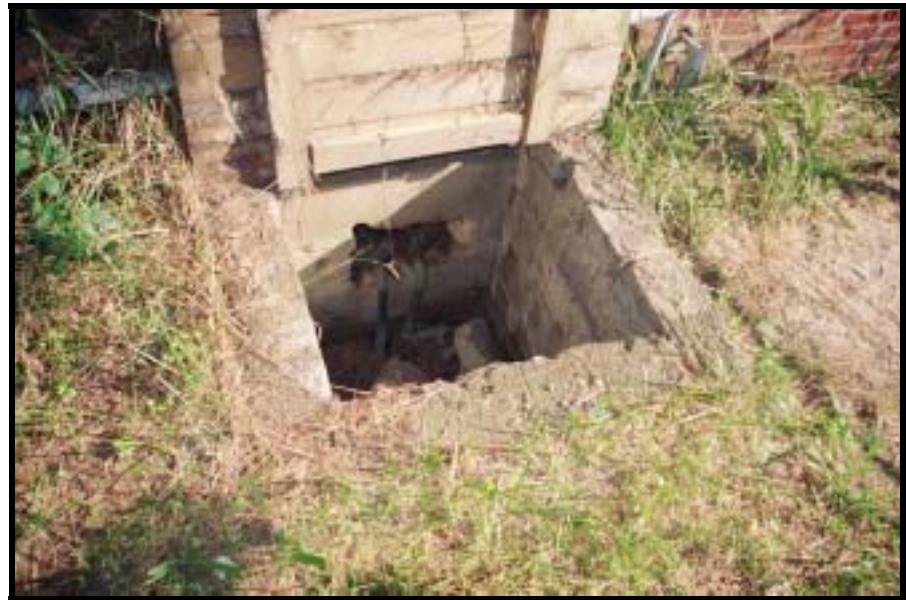
Figure 13. Plumbing access well located at south side of building.
