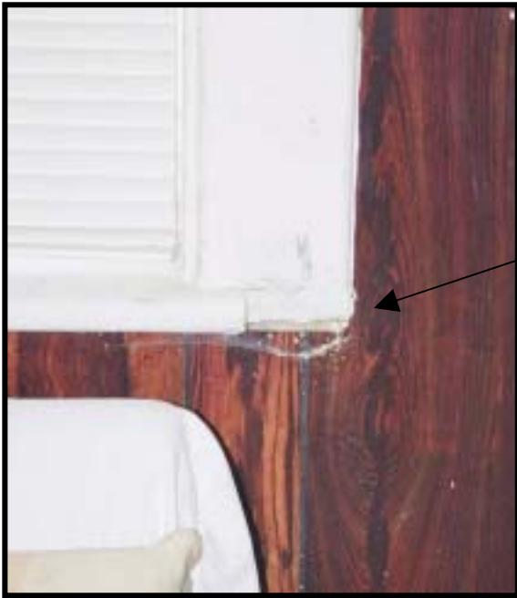
Figure 29. Detail of notch in stool of window W- 114 where original counter or desk may have butted into the east wall of room 103.
