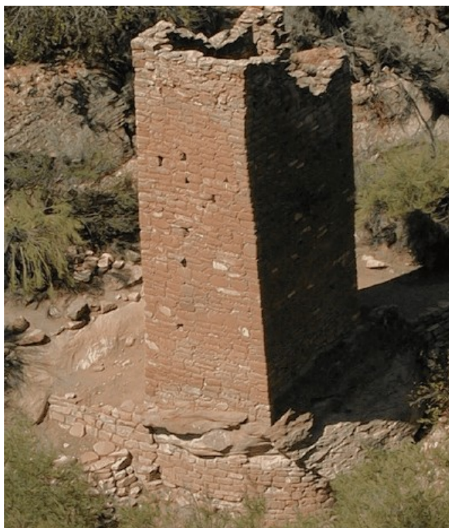
Photograph Caption: Square Tower, at Hovenweep National Monument. The tower was built on a slump block of Dakota Sandstone which is eroding due to the presence of a nearby stream. The stabilizing wall below the boulder was built by the National Park Service in 1960. (Photograph by Anne Poole, 2000).
