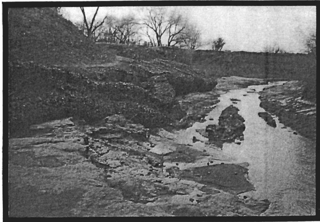
Photo 21: Continued failure of the gabion and channel incision, view downstream (May 1983), southwest.
