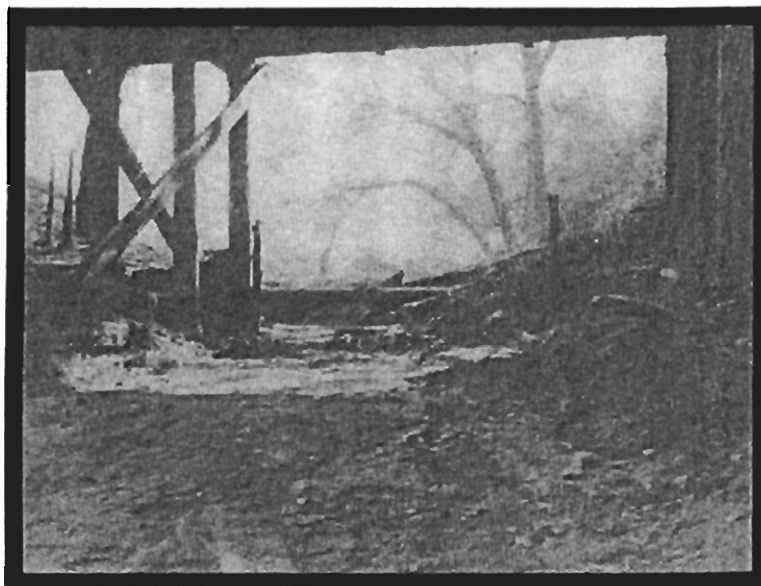
Photo 19: Headcutting (including undercutting of a utility line) in the Upper Tributary beneath the access bridge (November 1974).
