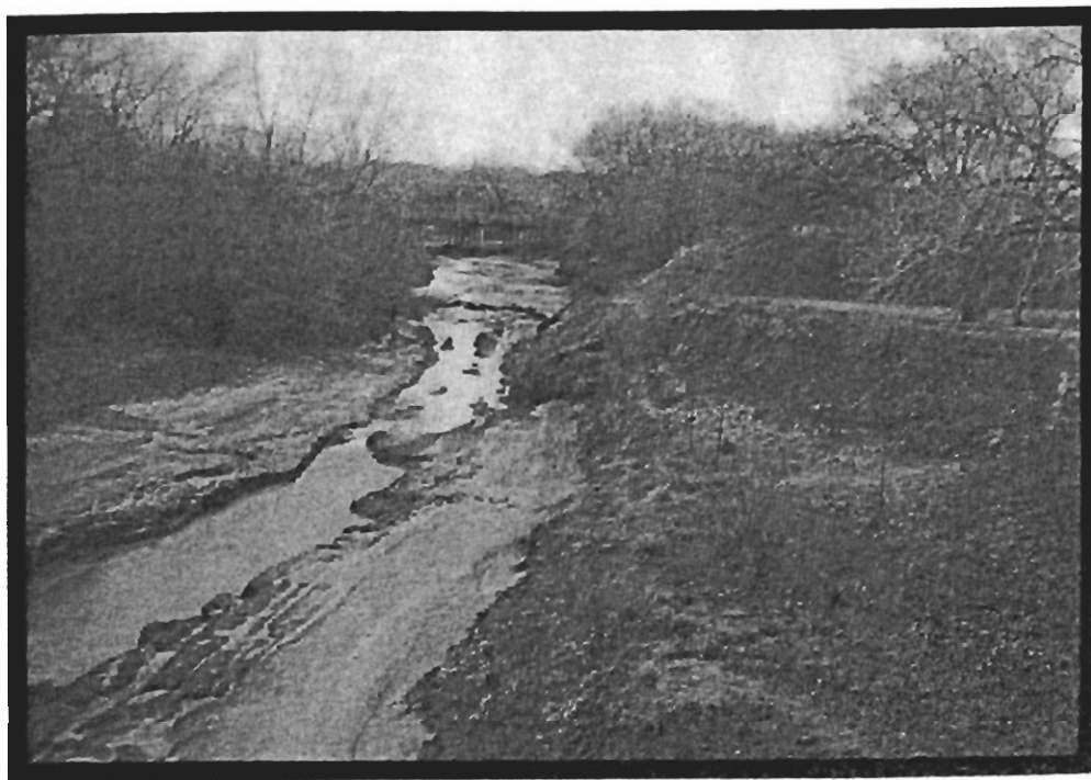
Photo 20: A view upstream from the Sand Dune Site showing the failing gabion, the highway bridge, and channel incision (May, 1983).
