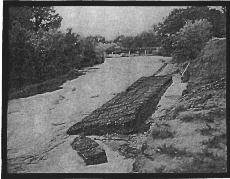
Photo 15: Close-up of subsidence of the engineering structure, due to undercutting, and the pulling away from the bank.
