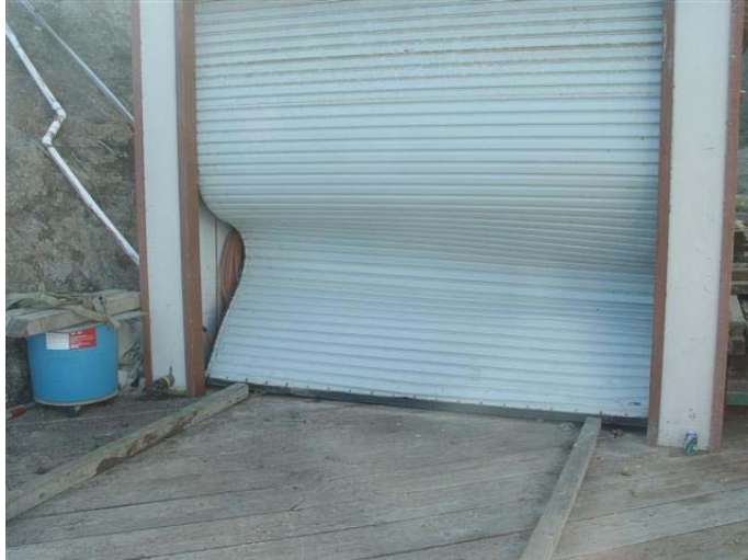
Figure 17. Wave damage to Santa Barbara Island Boathouse, November 2002.
