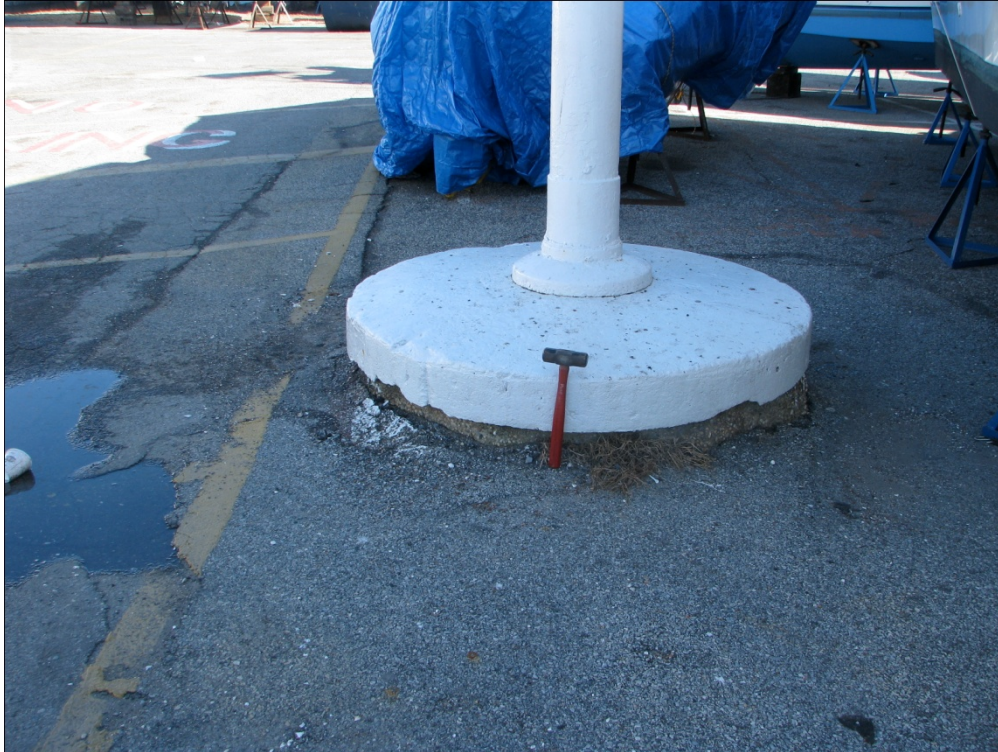
Figure 2. Lowering of parking lot surface relative to flag pole, 10-12 cm. March 24, 2009
