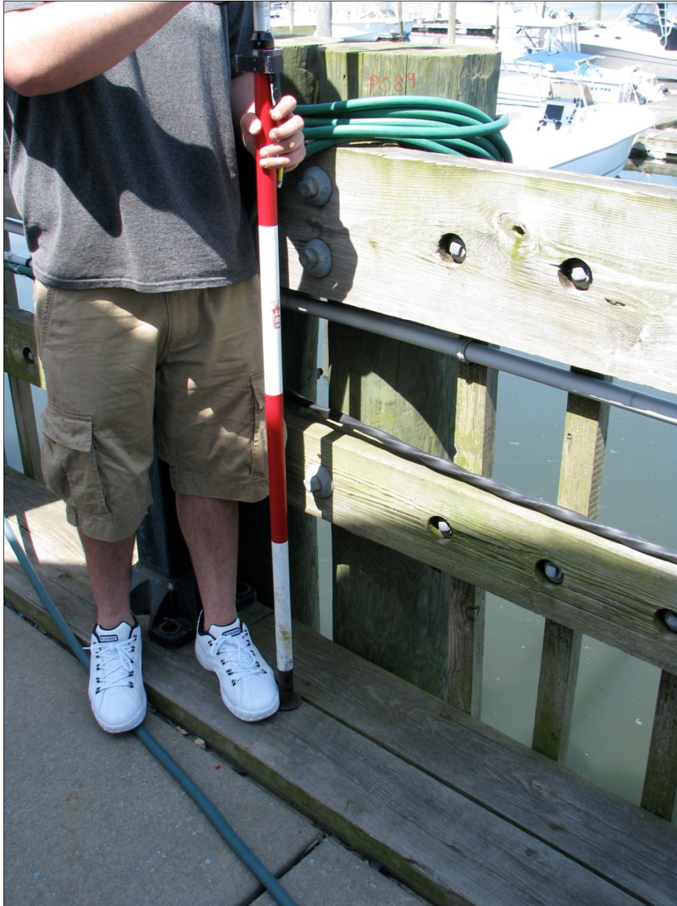
Figure 1. Lowering of the concrete surface adjacent to the marina bulkhead, 7-8 cm. May 24, 2010.
