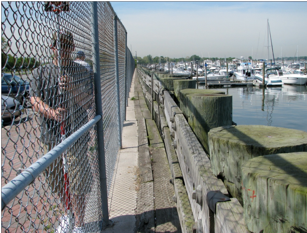
Figure 3. Shift of bulkhead and pilings into marina, less than 10 cm. northern end of marina. May 24, 2010.
