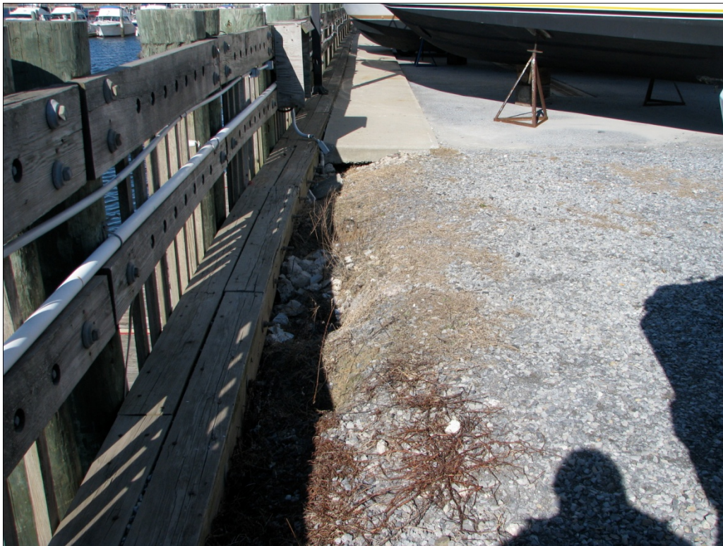
Figure 5. Sediment lost at inland margin of bulkhead, some gaps 10s of cm deep. March 24, 2009.
