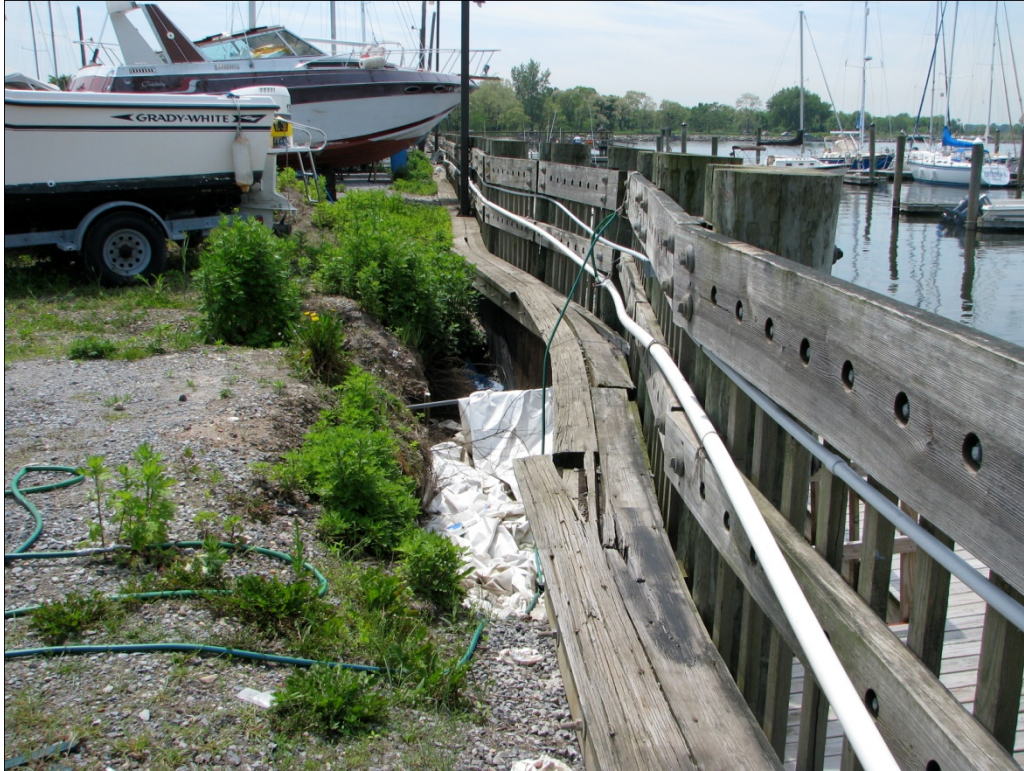
Figure 4. Major shift of pilings and bulkhead into marina, 25-30 cm, May 24, 2010.
