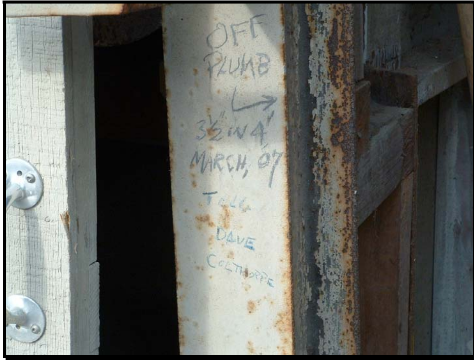
Figure No. 1292-6: Note on steel column recognizes the lateral movement of the frame.
