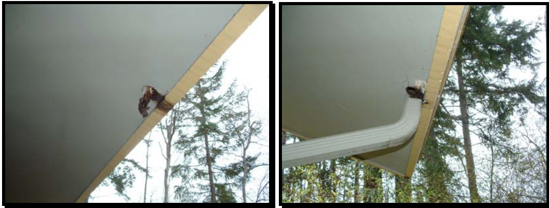
Figure No. 16-3: Deterioration of downspouts on west elevation
