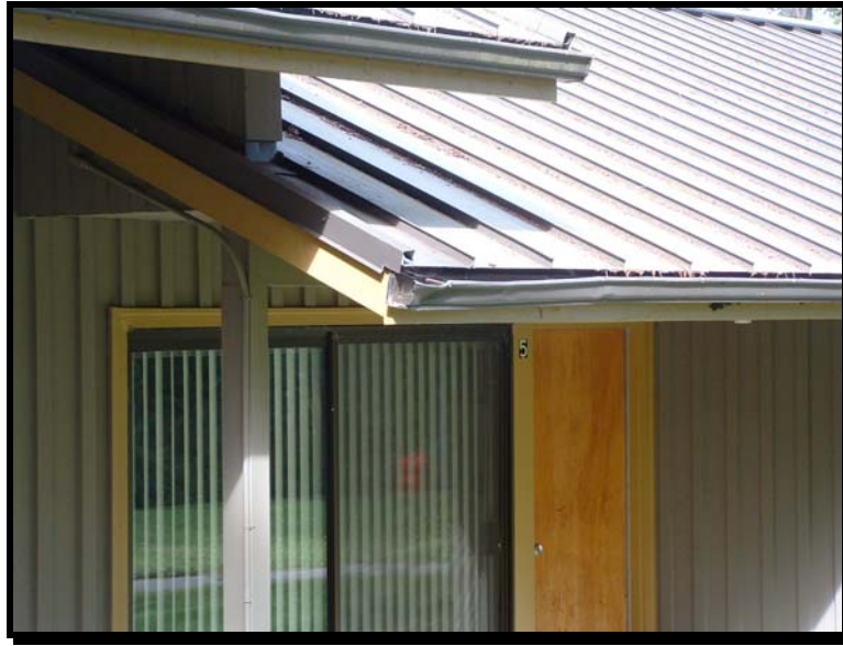
Figure No. 17-3: Existing gutter damage
