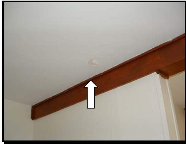
Figure No. 2-19: Plaster deterioration in the ceiling of kitchen hallway.
