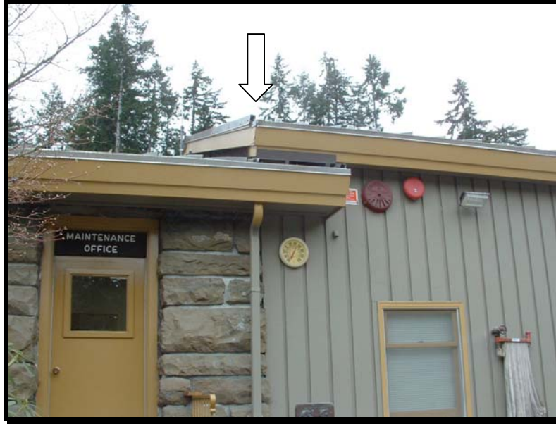
Figure No. 1000-9: Indications of fascia deterioration can be seen at the corner of the rake and eave.
