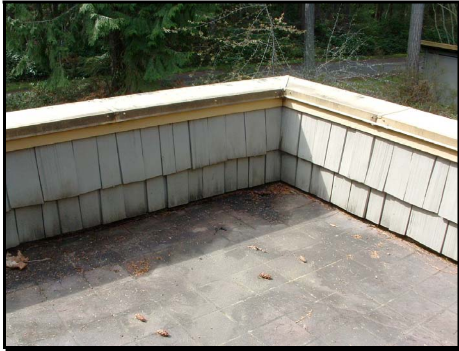
Figure No. 2-15: Quarry tile roof of sundeck; note overflow scupper has been covered.
