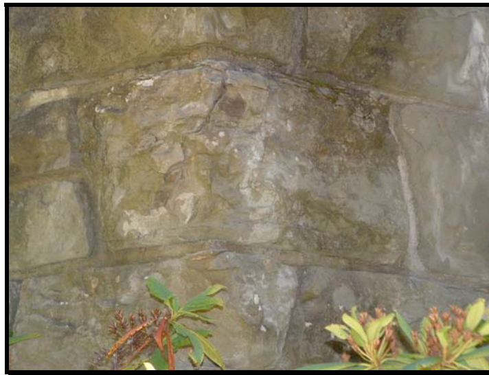
Figure No. 2-9: Surface deterioration on the chimney base.
