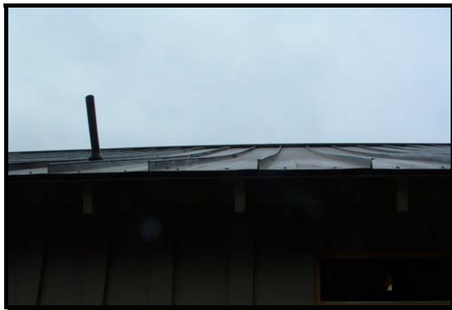
Figure No. 5-4:Roof deflection along the north slope
