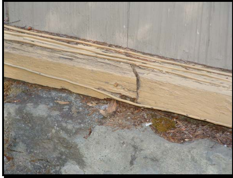
Figure No. 2-12: The foundation trim moldings is quite weathered and deteriorated.
