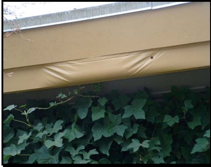
Figure No. 1000-7: Paint “bubble” on fascia full of water.
