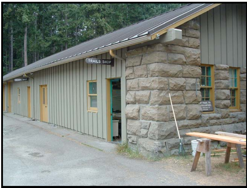
Figure No. 5-5: Test southeast outlooker for deterioration.
