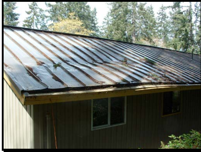
Figure No. 16-5: Southeast corner of roof eave showing current damage.
