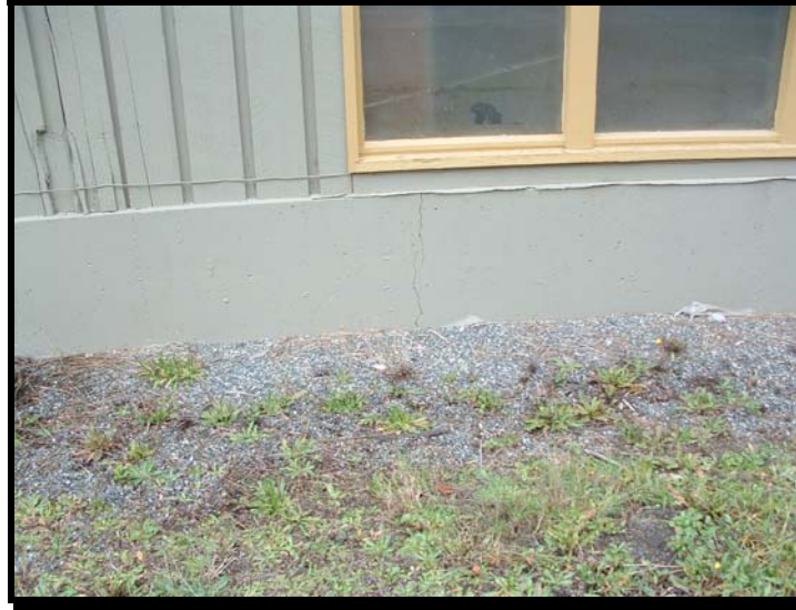
Figure No. 9-6: View of hairline crack under beneath the window
