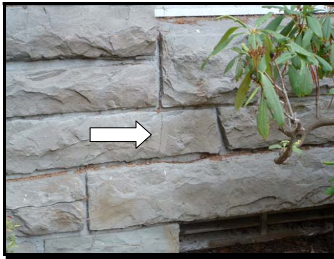
Figure No. 1-8: In the center of the picture there is a crack in the stone below the sill stone
