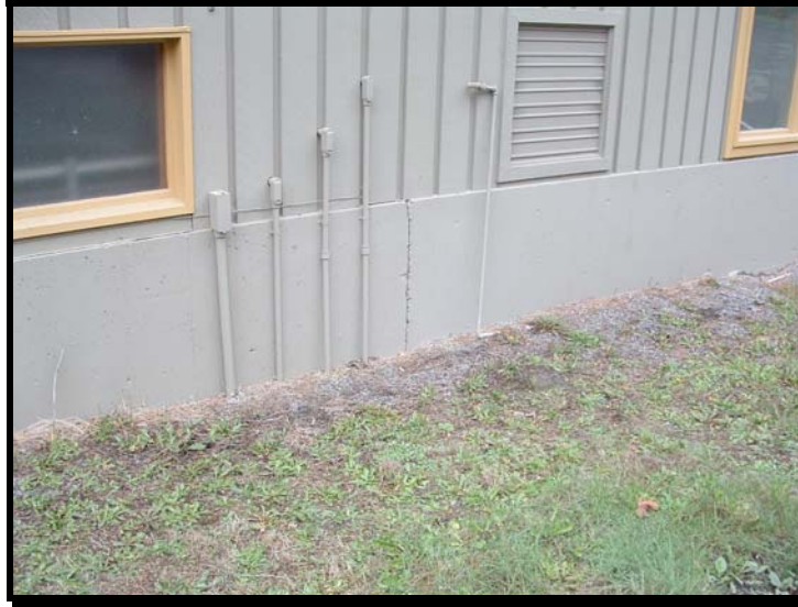
Figure No. 9-7: View of “cold joint”.
