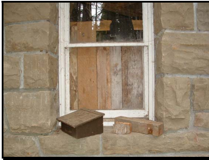
Figure No. 4-6: Missing glass in north window
