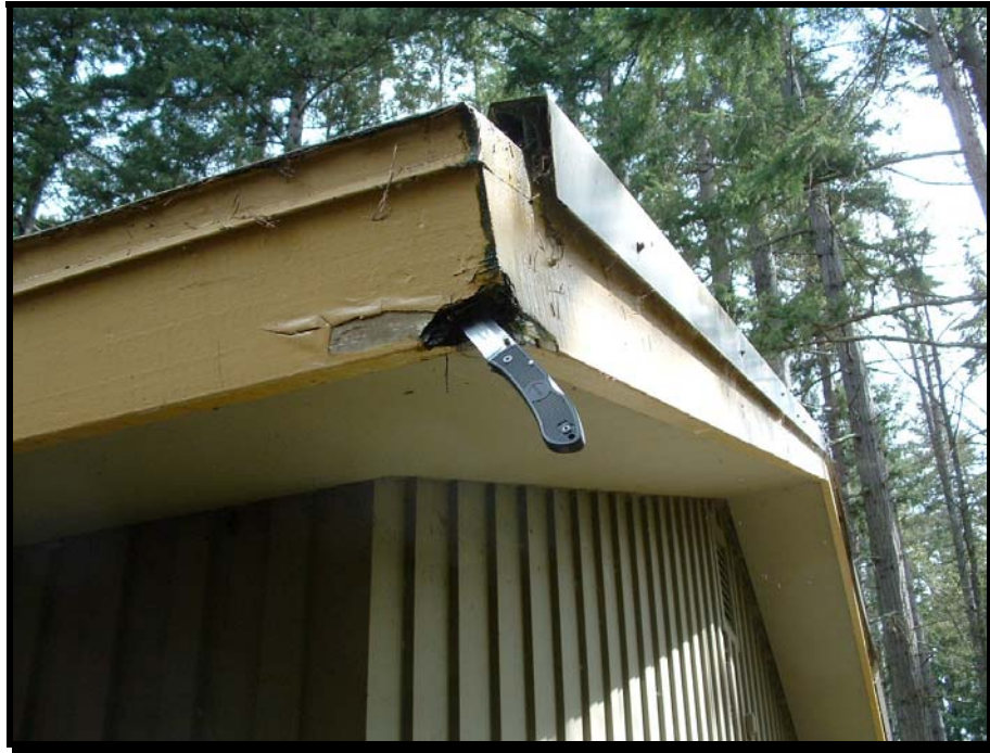
Figure No. 16-4: Southwest corner of roof eave showing current deterioration.
