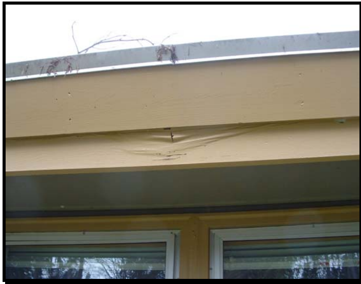
Figure No. 1000-8: Paint “bubble” on fascia that has broken.
