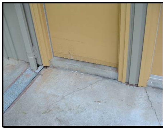
Figure No. 17-4: Delamination on exterior doors
