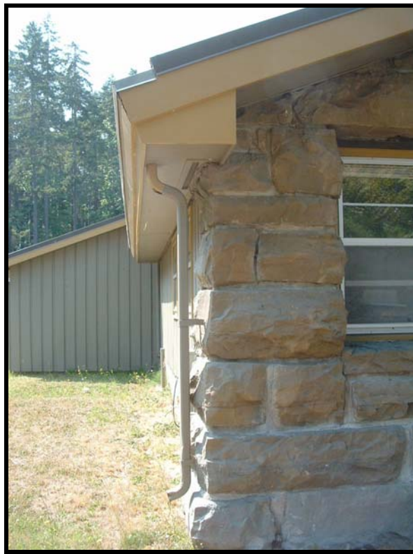
Figure No. 1000-5: Mortar cracking at southeast corner.
