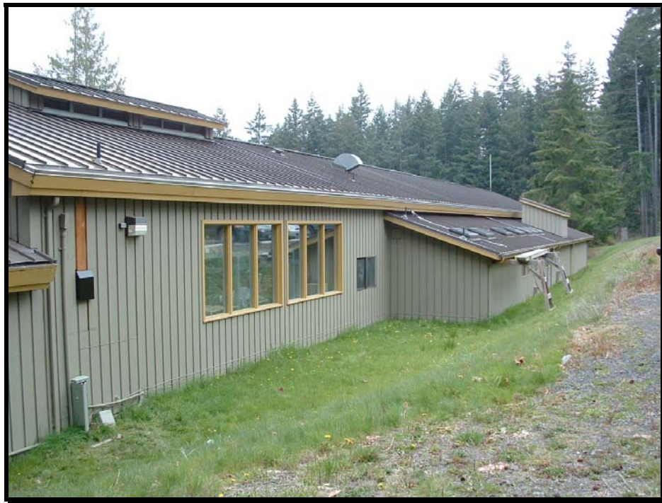
Figure No. 1000-4: At the rear of the building, the building had a grade apron to collect water from the above slope; this has been somewhat compromised by the rear shed addition.
