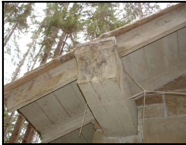
Figure No. 4-5: The false beam-ends are cracked and checked.
