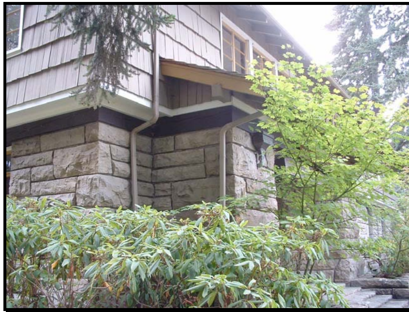
Figure No. 1-6: At the front entry, note abandoned leader box and new routing of downspout.
