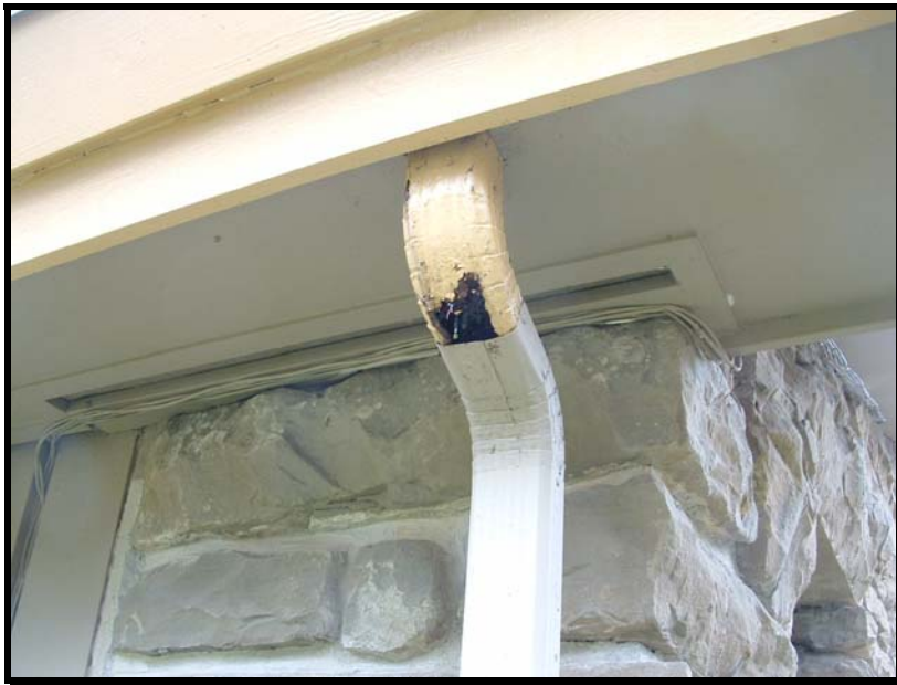
Figure No. 1000-10: Deterioration in the thru-eave downspout section.
