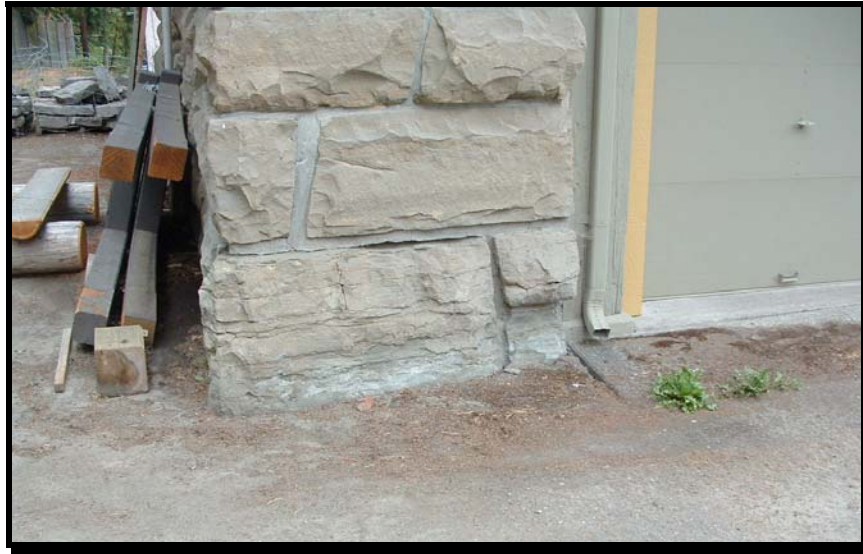
Figure No. 5-3: Southwest corner; the discoloration of the stone is from excessive moisture from the adjacent downspout; the weathering causes associated mortar cracking and bond loss.
