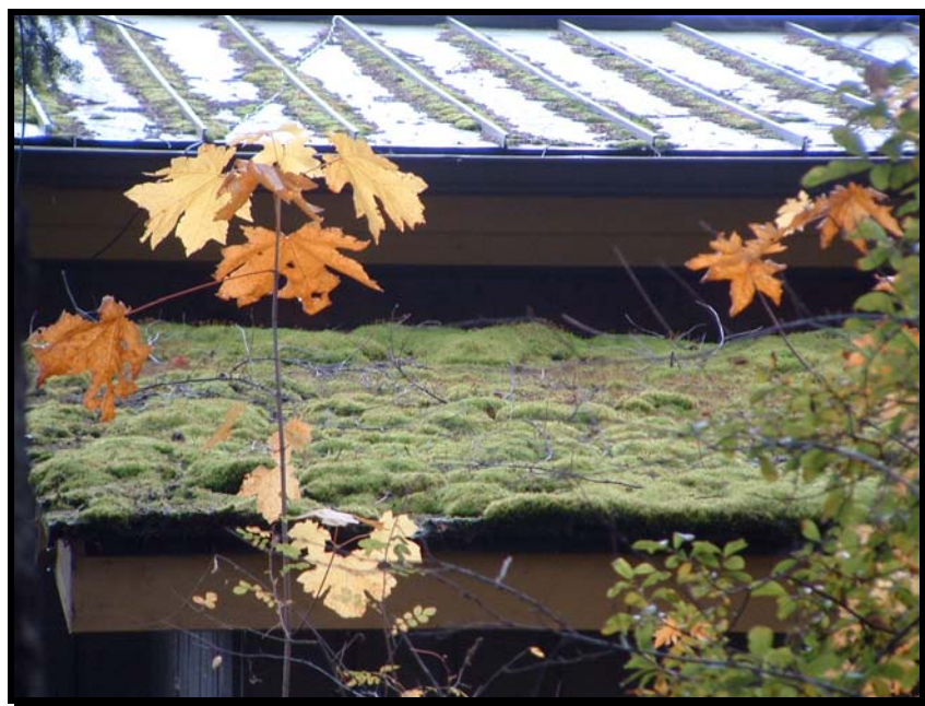
Figure No. 8-3: View of moss build-up on roof of rear ell
