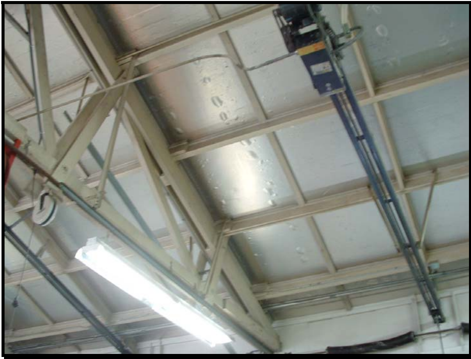
Figure No. 9-9: View of “bubbles” in insulation.
