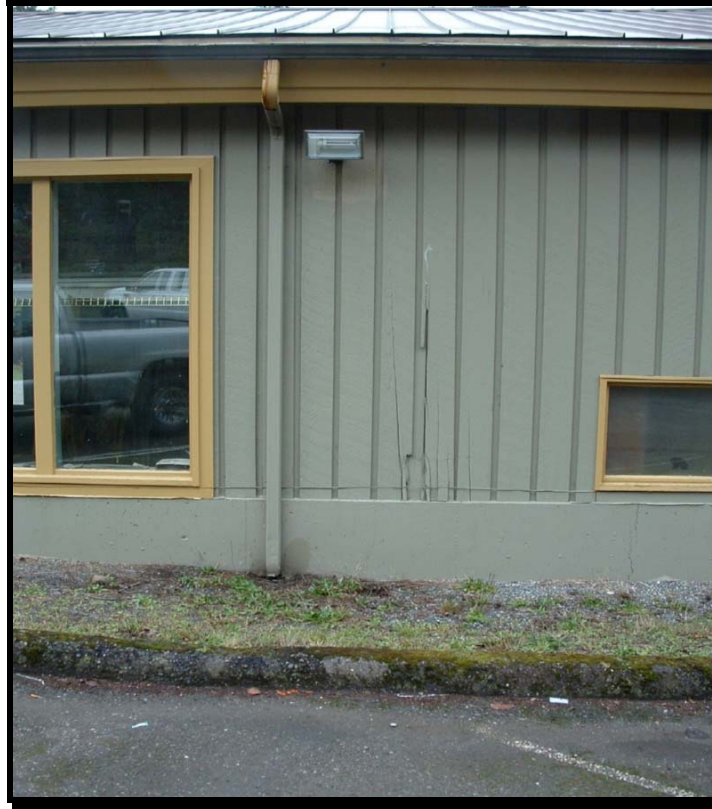
Figure No. 9-4: View of damaged siding
