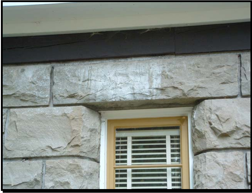
Figure No. 1-9: West elevation, staining of stone
