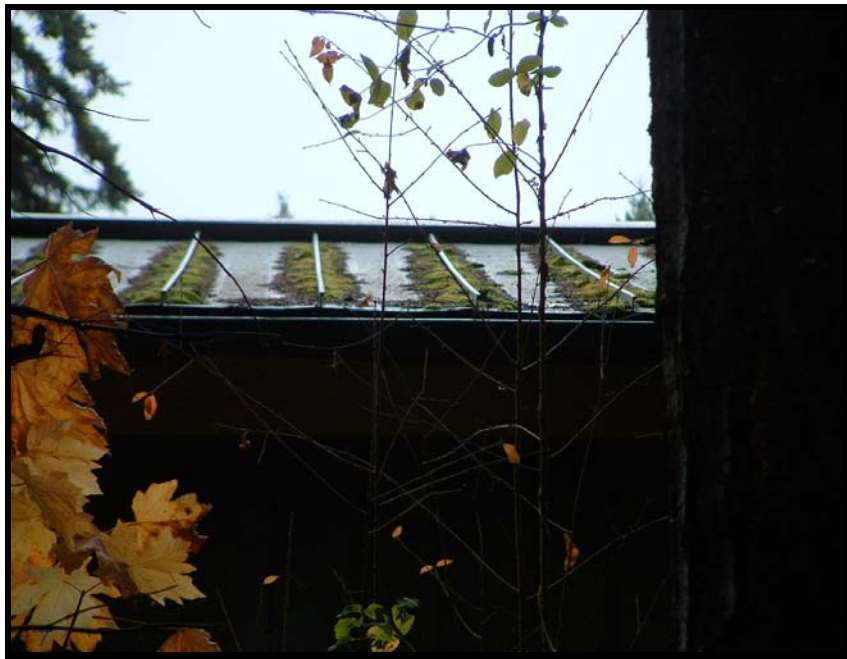
Figure No. 8-2: View north slope of roof; note build-up of moss and duff along standing seams and the deflection of the seams.
