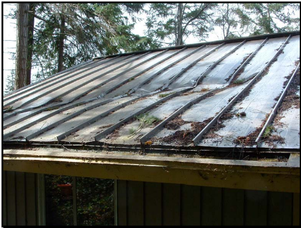
Figure No. 16-2: Southeast corner of the roof showing damage caused by tree fall.
