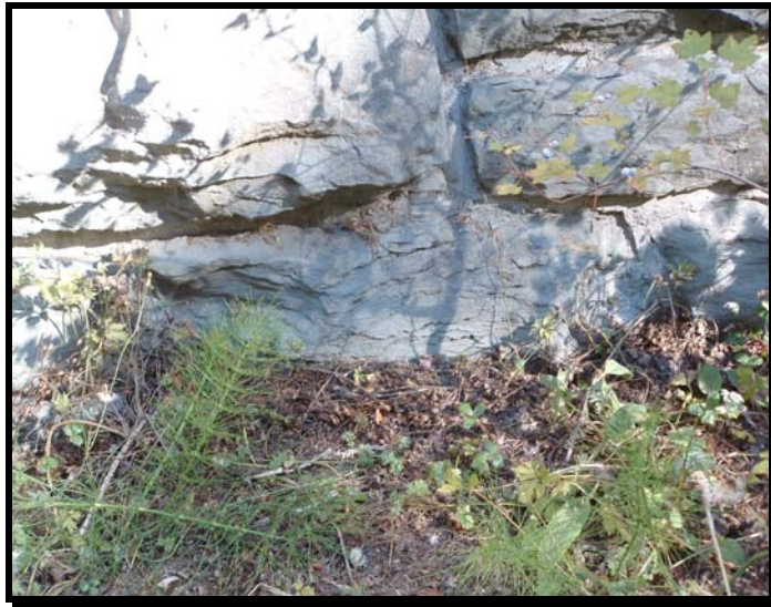
Figure No. 2-7: Veneer foundation stone deterioration
