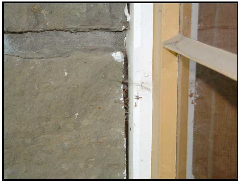
Figure No. 2-13: Note open joint at wood frame/stone interface.
