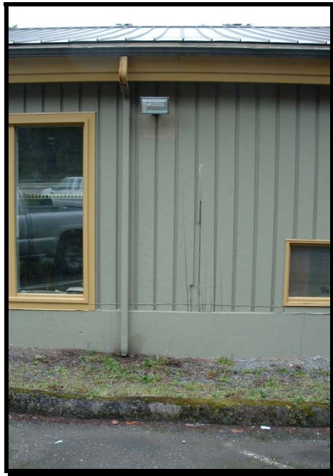
Figure No. 9-2: The central downspout on the south elevation is deteriorated at its base; note moisture absorption on concrete foundation.
