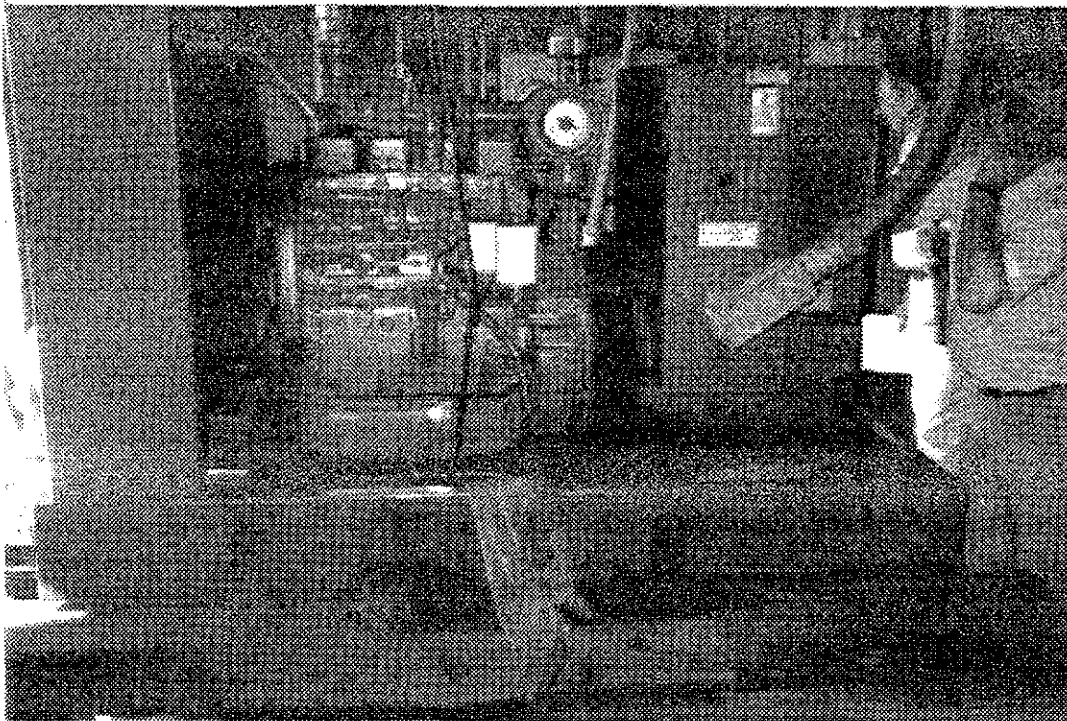
SHIP ISLAND North Generator Building East Generator November 8, 1994
