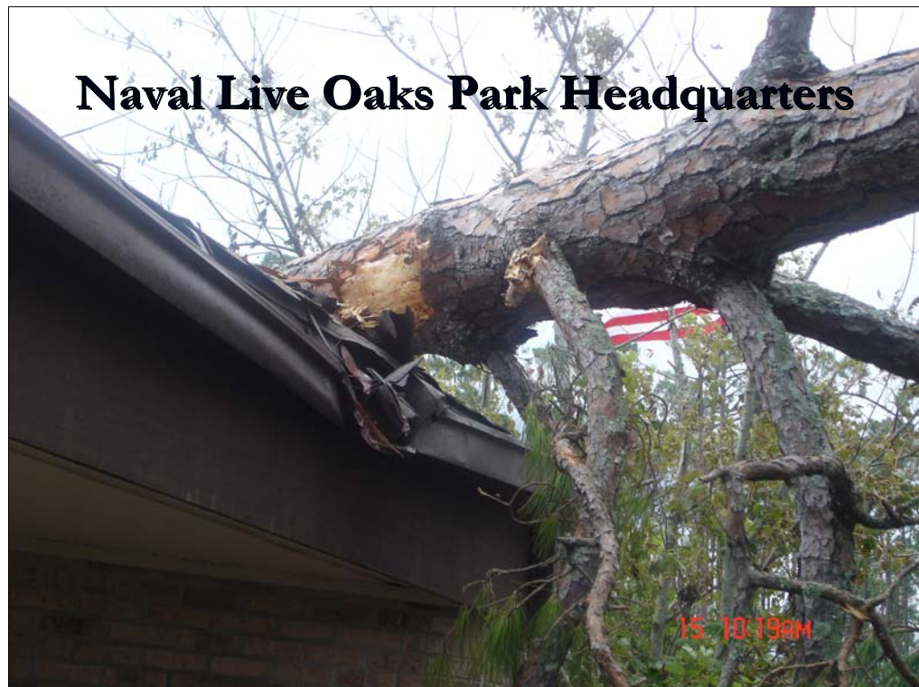
July 15 – Close-up photo of tree that fell on the corner of the park headquarters building
