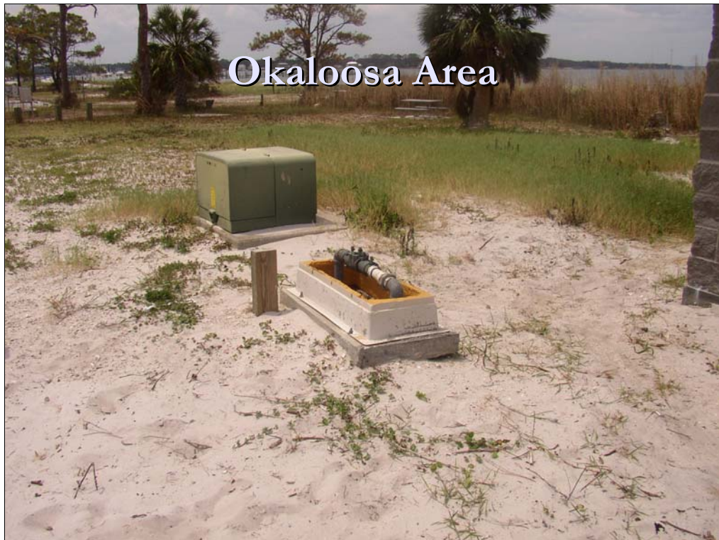
July 18 – Cover missing from water shut-off valves at Okaloosa Area.
