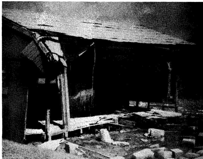
Residential Damage - Port Mansfield
