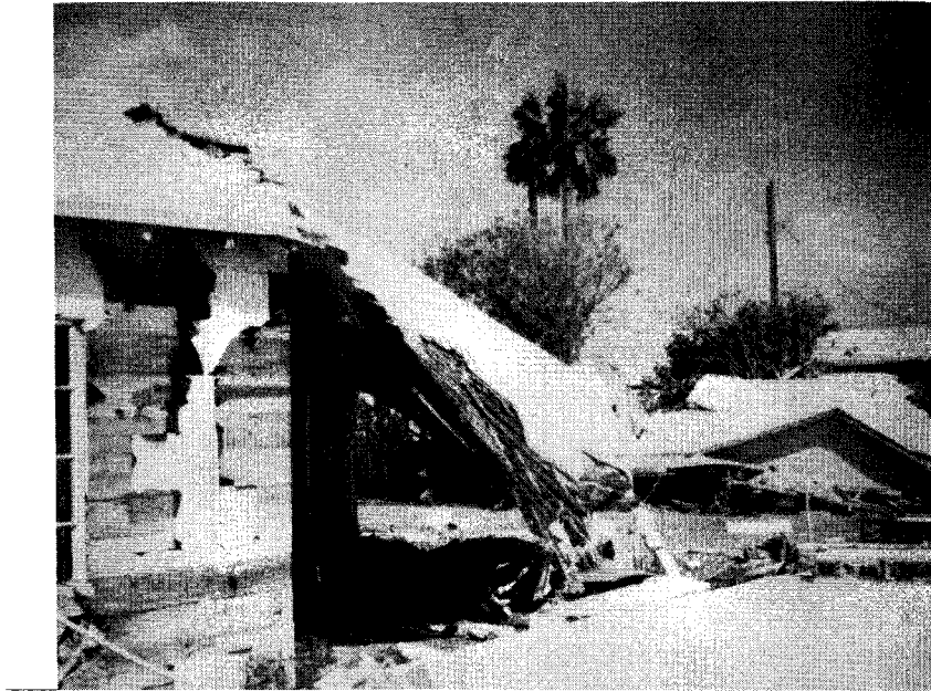
Residential Damage - Port Mansfield
