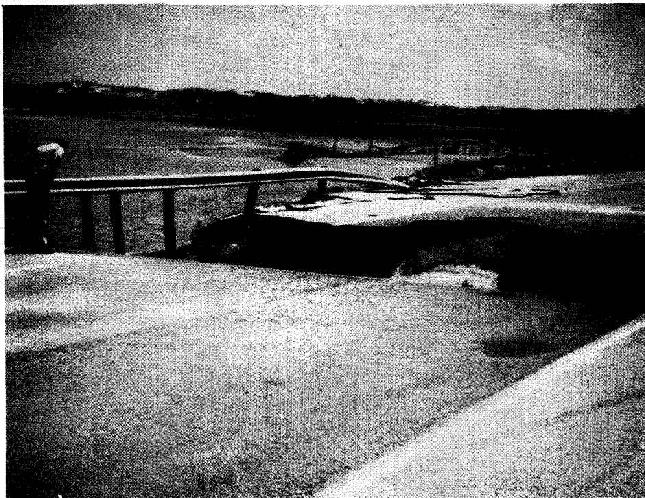
Road Damage - Mustang Island
