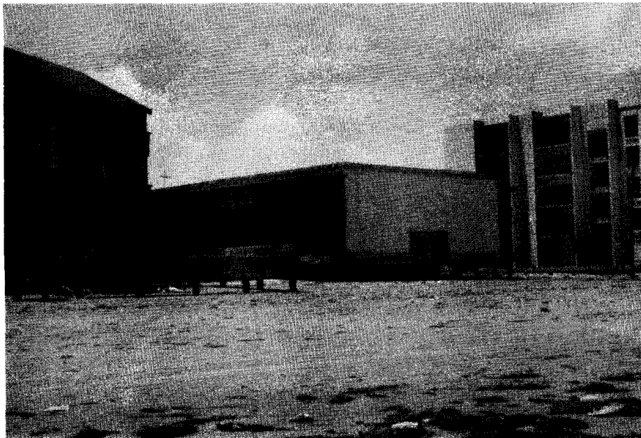
Undermining Damage - Port Isabel
