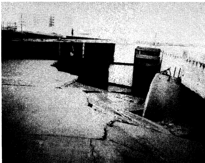
Seawall Damage - North Padre Island
