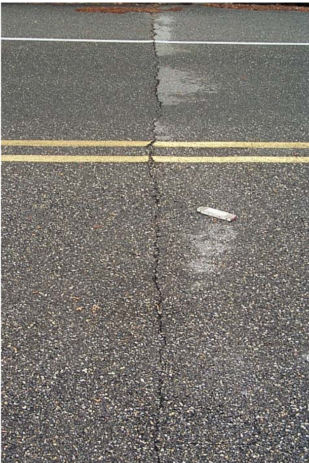
PHOTO #4 - TRANSVERSE CRACKING OF ASPHALT AT SOUTH APPROACH (PHOTO FROM 3/20/2001 INSPECTION)
