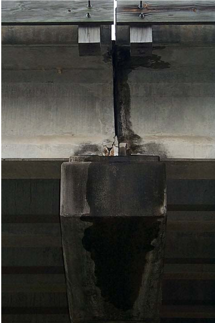
PHOTO #5 - NORTH PIER, EAST SIDE; NOTE MINOR SPALL AT END OF BEAM AND STAINING OF PIER CAP (PHOTO FROM 3/20/01 INSPECTION REPORT)
