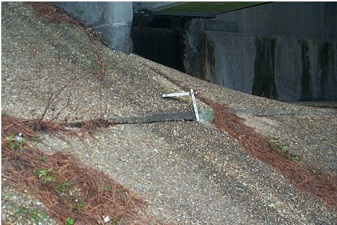
PHOTO #6 - SETTLEMENT OF SLOPE PAVING AT EAST SIDE OF SOUTH ABUTMENT (PHOTO FROM 3/20/01 INSPECTION REPORT)
