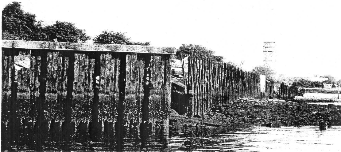
Figure 6. This corner of the shoreline is an erosional hot spot due to the high energy of the corner design. The failure of the SSP bulkhead allowed erosion of the backfilled area behind the bulkhead.
