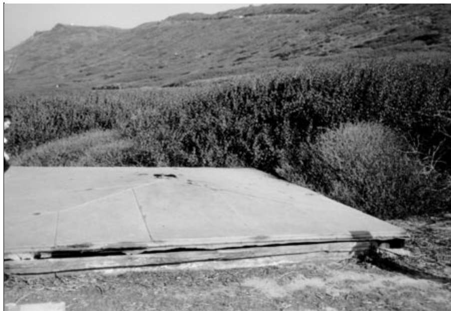
Figure 39. Deteriorated wood curb at Searchlight Shelter No. 15.
