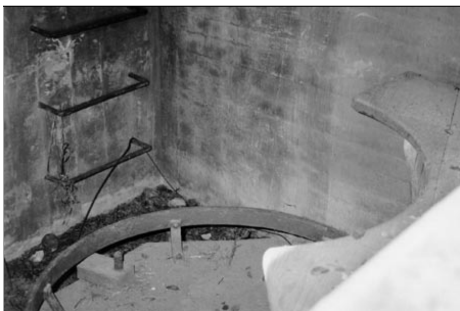
Figure 19. Embedded metal ladder rungs provide access from the hatch opening above.
