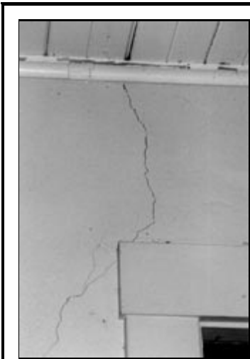
Figure 31. Concrete cracks at Army Radio Station headers.
