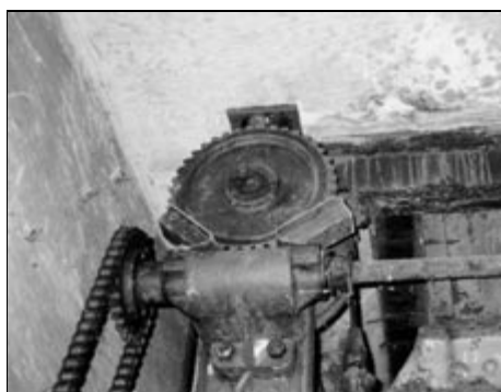
Figure 36. Coating failure and corrosion at Searchlight Shelter No. 15.
