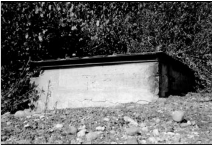
Figure 32. Concrete cracks at Base of Battery Calef & Wilkeson Base-End Station hatch.
