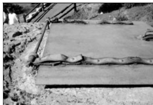
Figure 37. Metal corrosion of hatch at the Battery Commander Station, Battery Humphreys.
