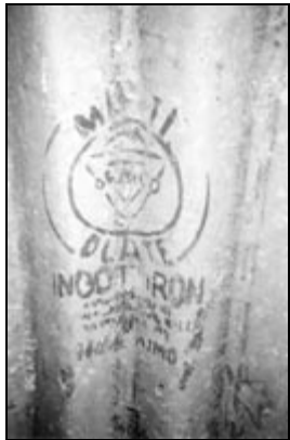
Figure 42. Graffiti on corrugated metal at Battery Point Loma Bunker Complex.
