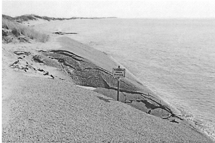
Figure 10. An asphalt bulkhead that lines a section of the foreshore at Herring Cove Beach is failing and may be unsafe.
