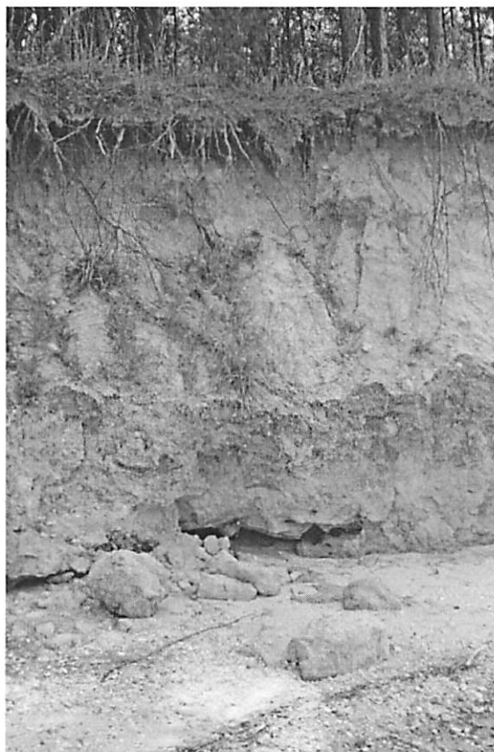
Figure 20. Bluffs are actively eroding through processes of undercutting and subsequent slumping. This photo shows the undercut bluff as well as debris (boulders on beach) left from an earlier failure. The numerous tree roots exposed at the top edge of the bluff are evidence that the bluffs are actively eroding.
