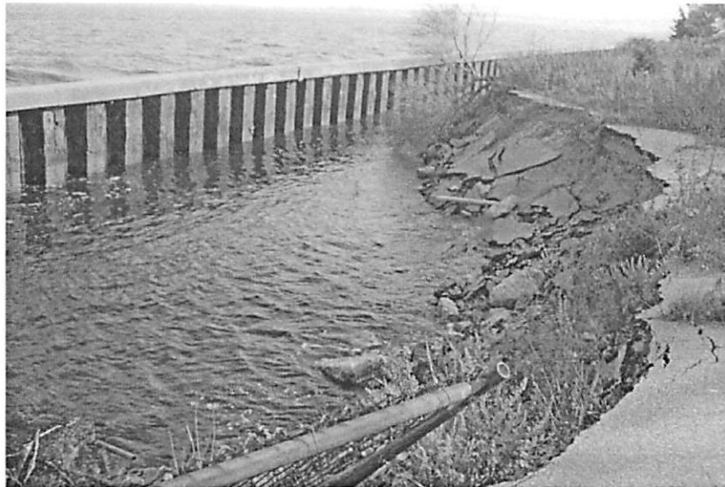
Figure 14. Erosion caused by scouring behind bulkhead at Floyd Bennett Field.
