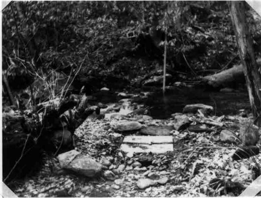
INTAKE STRUCTURE FOR COSBY CAMPGROUND WATER SYSTEM ON COSBY CREEK
