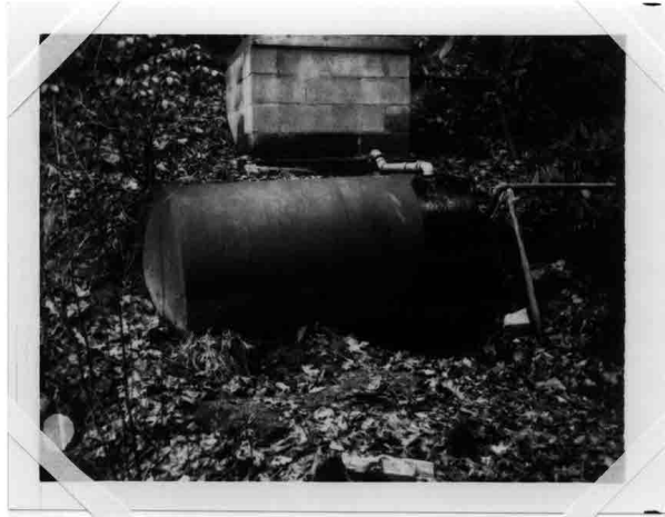
A 500 GALLON STEEL TANK RESERVOIR FOR RESIDENCE AT OLD OCONALUFTEE AREA THE CONCRETE BLOCK HOUSE IN UPPER PART OF PHOTO IS AN ATTEMPT AT A SAND FILTER FOR THE SYSTEM.
