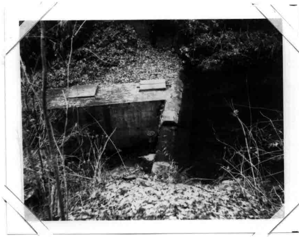
WATER INTAKE STRUCTURE, INCLUDING CONCRETE DAM AND SAND FILTER SERVING TREMONT RANGER STATION
