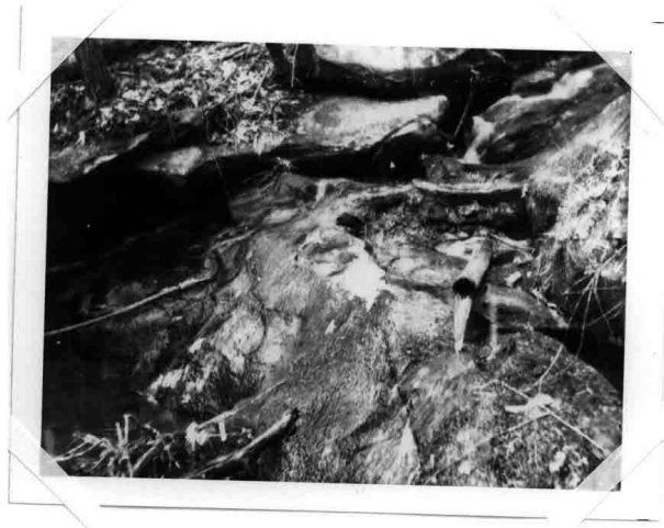
Left: Intake Structure Serving the Water System at Twentymile Ranger Station
