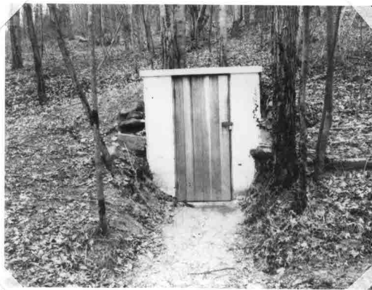
CHLORINATOR HOUSE HOUSING AN AERO-FEED CHLORINATOR AND A WATER METER
