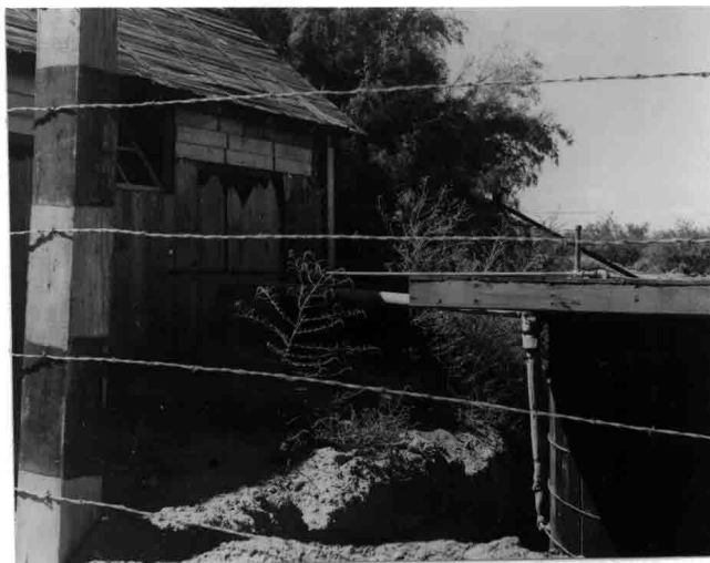
No. 2. Water flows by gravity to this wooden stave storage tank. It was necessary to sink the tank below grade to obtain proper gradient for pipe line.
