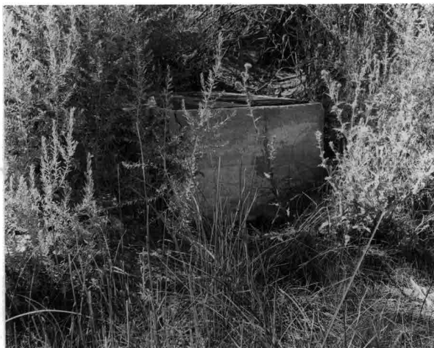
No. 1. Spring box around Angell Spring. Box is approximately 3' x 4' x 6'-0". Pickup line at box is about 5" pipe with welded joints. An overflow exists so that only a portion of the water is collected in the pipe.
