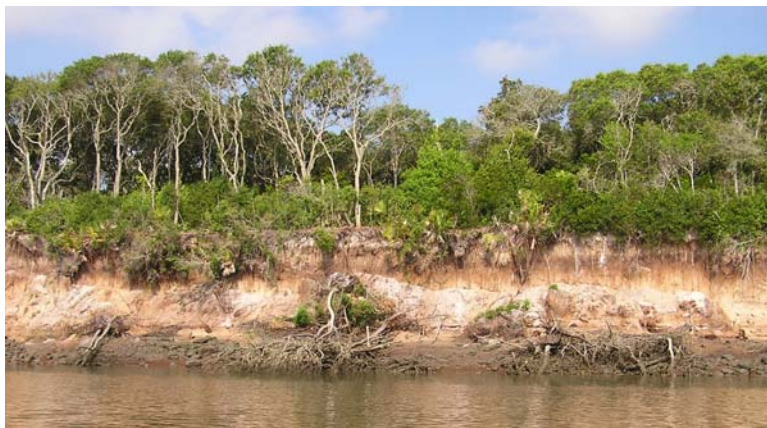
Figure 11 Half Moon Bluff on Simpson Creek showing tidal current-induced erosion.
