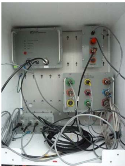
Figure 15. Inside of instrument enclosure just before departure (Fourpeaked RAWS).
