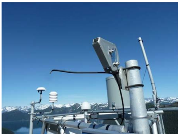
Figure 27. Broken GOES antenna (McArthur Pass RAWS).
