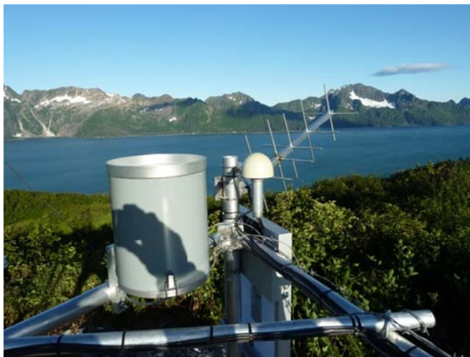
Figure 36. Rain gauge, satellite antenna, and GPS antenna (Pedersen Lagoon RAWS). Barb wire was mounted above the sensor cables on the southern frame section in order to mitigate damage from wildlife (bears).
