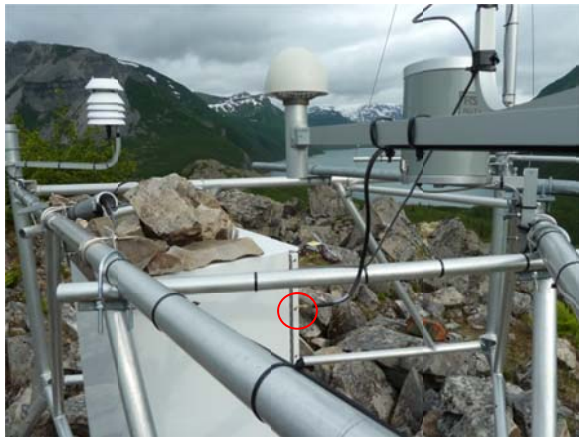
Figure 16. The GPS antenna cable was cut (circled) and there were bite marks on the GPS antenna (Hickerson Lake RAWS).
