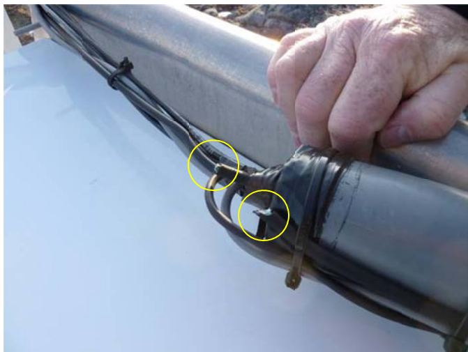
Figure 22. Severed snow depth sensor cable (McArthur Pass RAWS).
