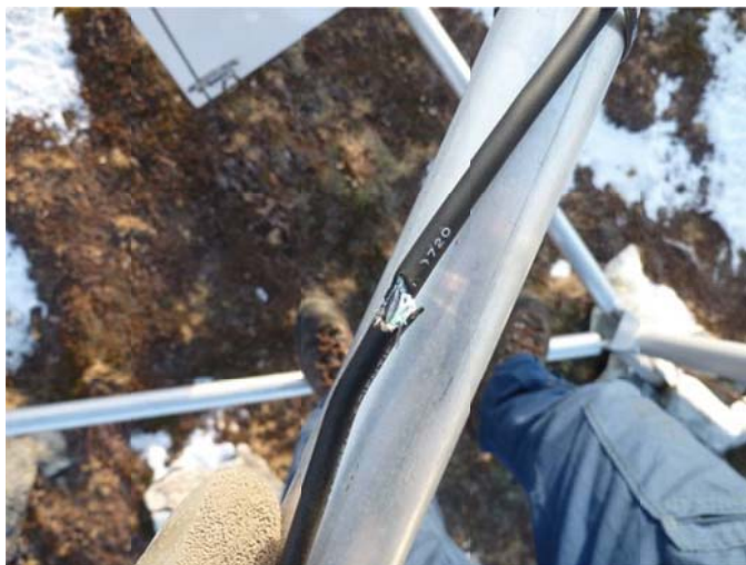
Figure 23. Damaged snow depth sensor cable (McArthur Pass RAWS).
