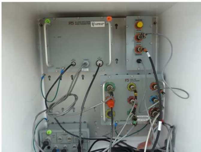
Figure 44. Inside of instrument enclosure photographed just before departure (Pfaff Mine RAWS).
