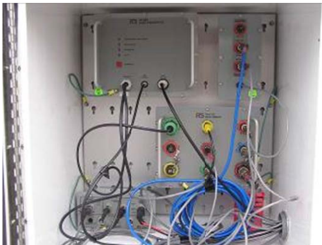
Figure 8. Inside of instrument enclosure photographed just before departure (Contact Creek RAWS).
