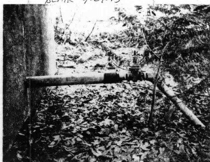
3" DISCHARGE FROM CISTERN
