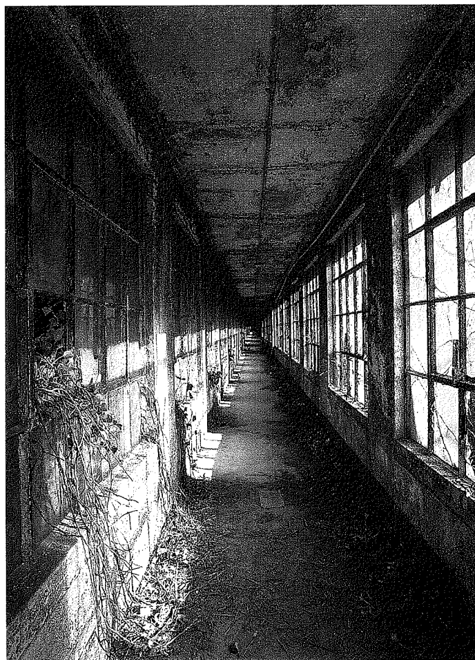
Many of the irreplaceable resources the parks were established to protect are vanishing. The hospital and quarantine wards on South Ellis Island are falling into ruin and closed to visitors because they are unsafe.
