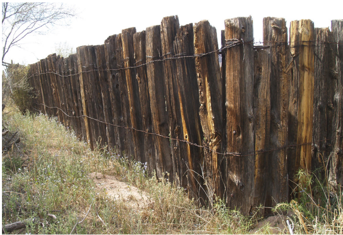
Figure 25: Stockade type fencing made from closely spaced timbers strung with barbed wire. Even though these posts have been treated with creosote, many have rotted off below grade causing sections of this type of fence to collapse. Photo: Randall Skeirik, NPS
