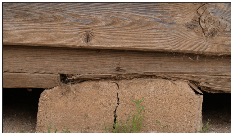
Figure 13: Along the north elevation of the hay barn, the 2x6 sill plate of the wall is severely deteriorated. This photo shows a point at mid-span where the plate is completely crushed where it sits on a concrete foundation block.
