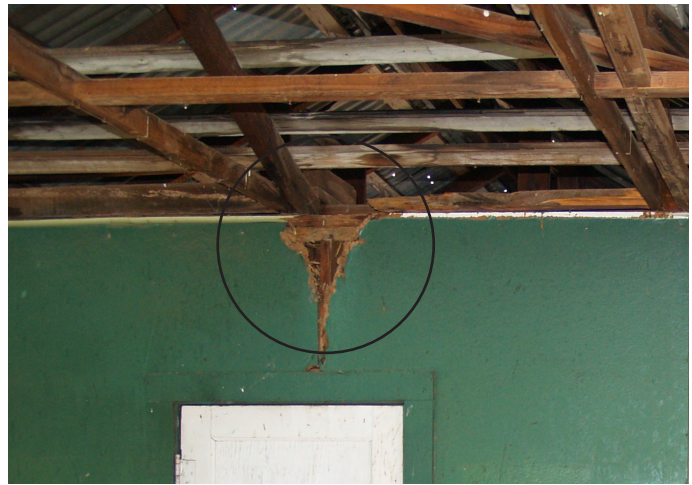
Figure 16: Area of the top plate of this wall has suffered termite damage at the point where it carries one of the roof rafters.
