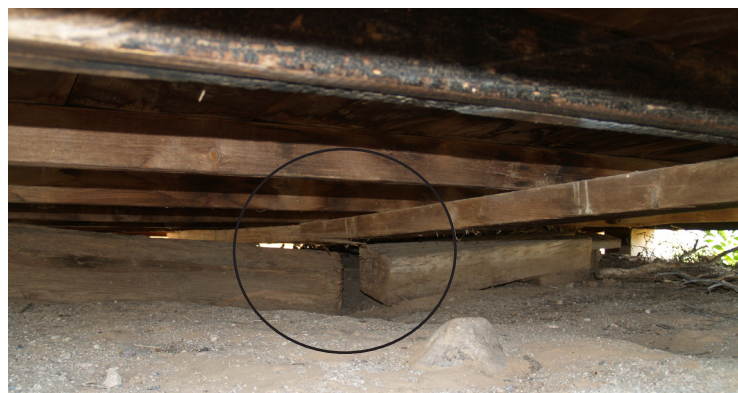
Figure 7: The longitudinal beam in the floor of the Bunkhouse is cracked. Timber supports were added some time in the past, but have been displaced.
