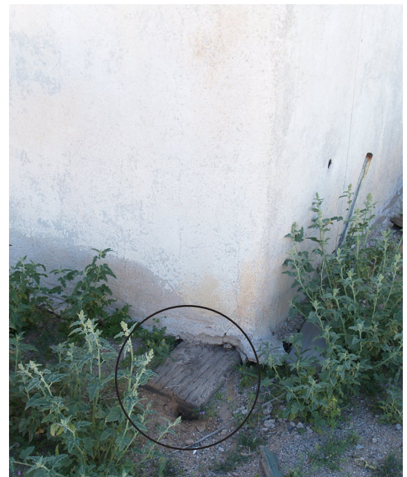
Figure 15: The timber footing projects out beyond the northwest corner of the building, the only place where it can be observed without excavation. Photo: Joe Tuomey, NPS
