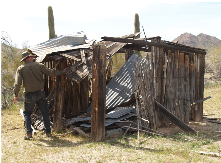
Figure 4: Jake Barrow, VT exhibit specialist inspecting the Ocotillo Shed. Actually constructed of saguaro ribs strung between railroad tie posts, this small structure needs immediate treatment to prevent collapse.
