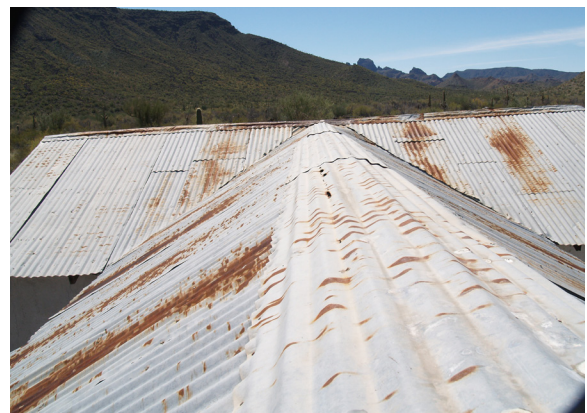
Figure 17: Nail hole patterns strongly suggest that the corrugated metal roofing on the Ranch House has been reused. Although it shows numerous rust patches only area has rusted through at this time.
