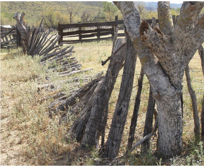
Figure 23: Stockade type fencing made from closely spaced mesquite posts strung with barbed wire. As with other fence types that use mesquite posts, many of the posts have rotted off below grade causing the fence to collapse. Photo: Randall Skeirik, NPS
