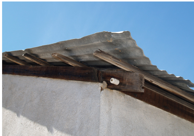
Figure 18: Deterioration of the purlins at this corner has allowed the nails that attach the roofing to pull out. The wind has caught this corner and is working more nails loose. Without reattachment, this section of roof will soon fail.
