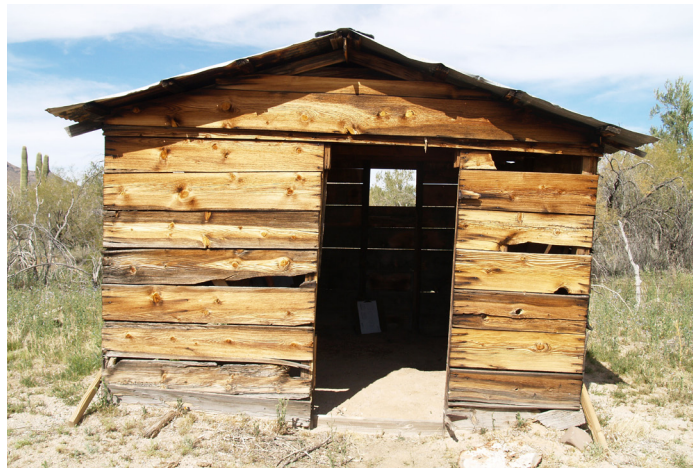
Figure 10: The Tack House is an important component of the ranch complex. Constructed with posts buried directly into the ground, the bottom ends of those posts have completely deteriorated.
