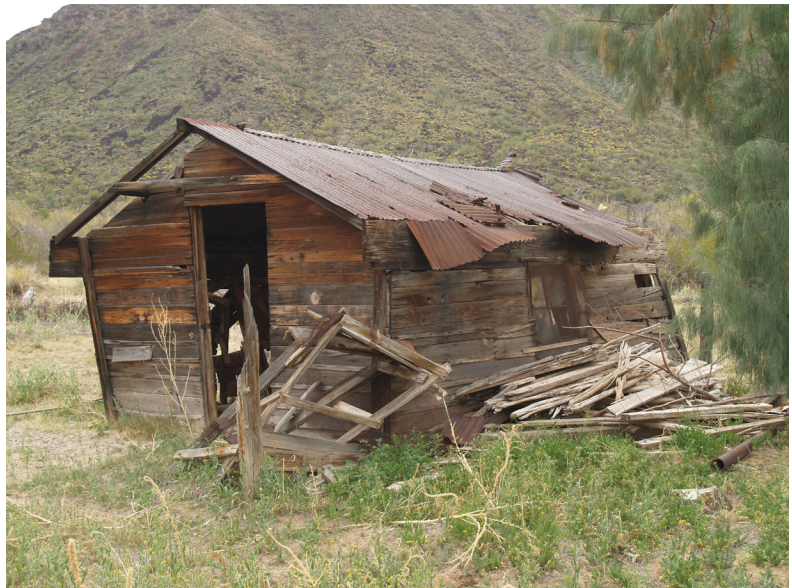
Figure 1: Front view of Chico's House (the Small Residence) showing how the structure is leaning to the left. Without rapid intervention, this building will collapse.
