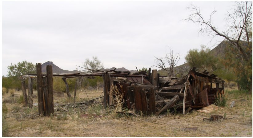
Figure 3: The Blacksmith Shop with the ramada shown to the left. This building has suffered significant deterioration over the past two years, but has not yet reached the point where it cannot be preserved. Photo: Randall Skeirik, NPS
