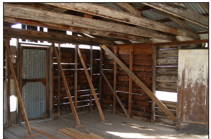
Figure 12: The gable-end walls of the Hay Barn have been braced because the wall's top plate and the tie to the bottom chord of the rafter are structurally inadequate. This temporary bracing should be removed and replaced with a more permanent and aesthetic solution.
