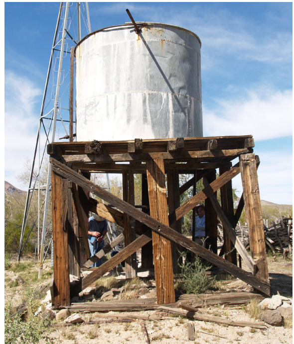
Figure 27: Water tank associated with Windmill Number 2. Note that the sill beam at the bottom front is badly deteriorated. This deterioration has allowed the support frame to wrack and has required the installation of additional diagonal bracing. Because the tank no longer holds water, the danger of collapse is small, nevertheless, the deteriorated framing members should be repaired or replaced.
