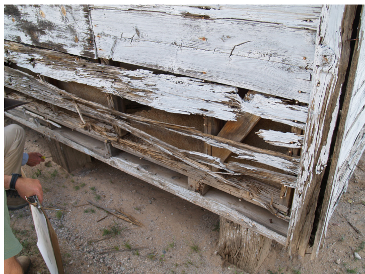
Figure 8: Some sections of the wood siding on the Bunkhouse have suffered severe termite damage. Replacement of this material may be desirable in the long-term, but it is not a high priority.
