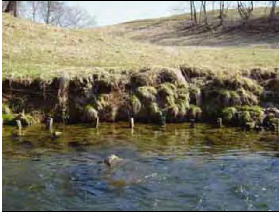
Erosion Location 23 (February 20, 2004)
