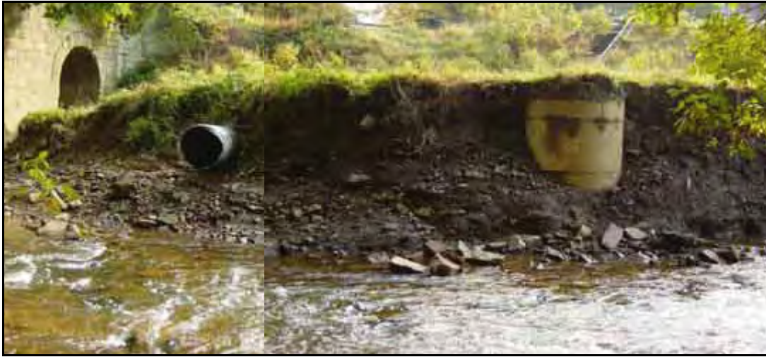
Erosion Location 1 (November 1, 2003)
