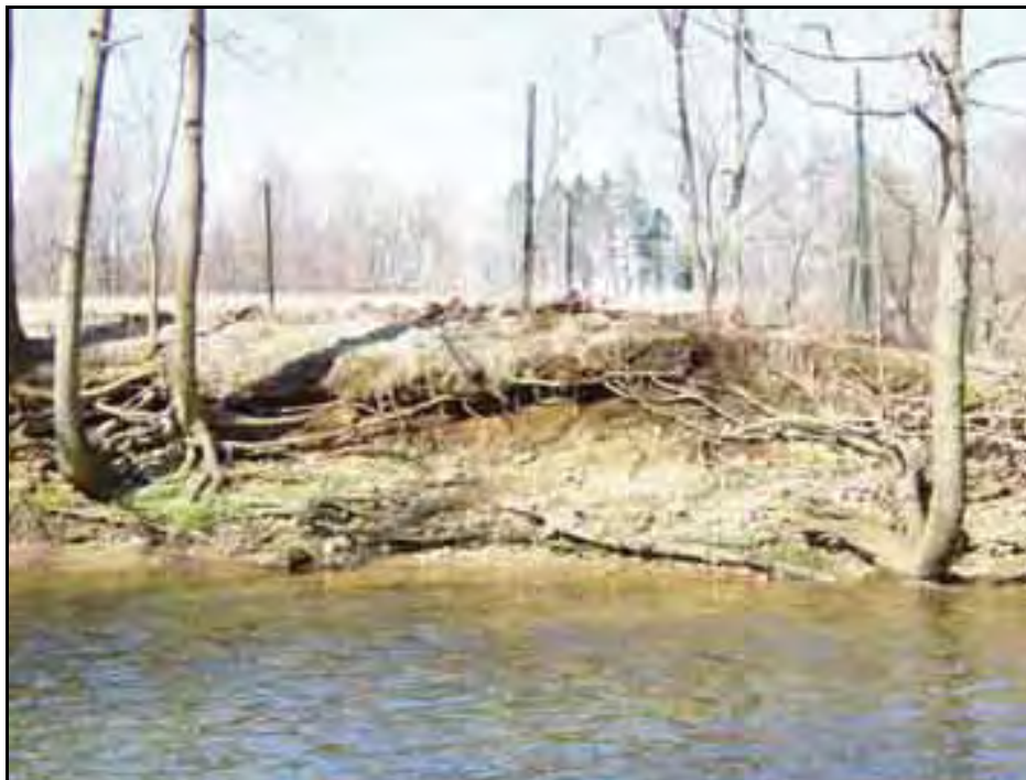
Erosion Location 28 (February 20, 2004)
