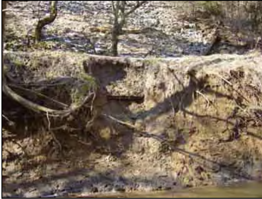
Erosion Location 17 (December 20, 2003)
