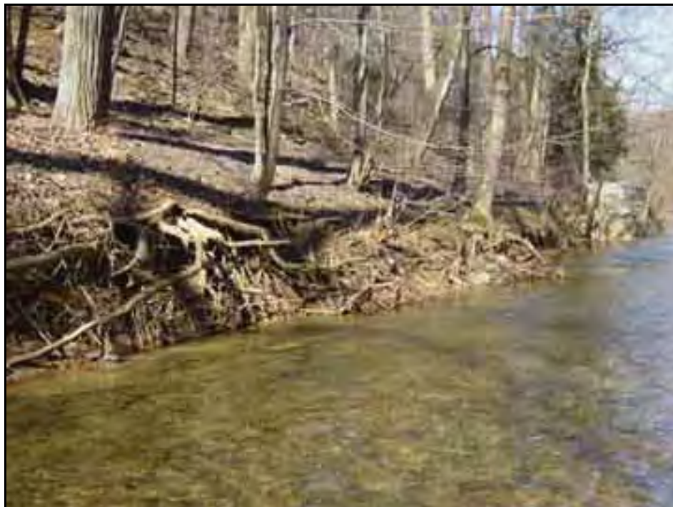
Erosion Location 18 (December 20, 2003)
