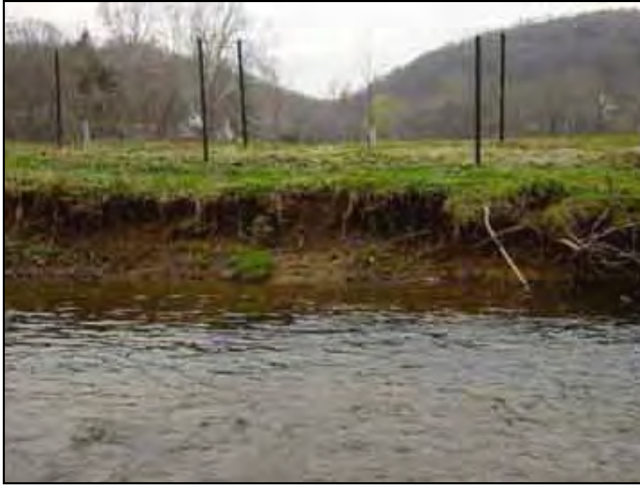
Erosion Location 31 (April 3, 2004)
