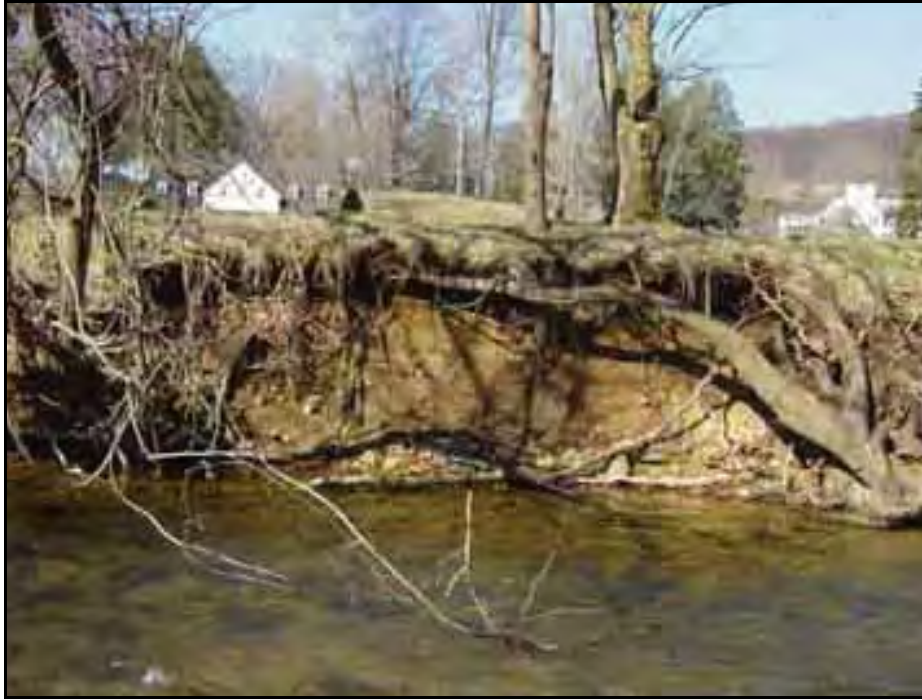
Erosion Location 25 (February 20, 2004)
