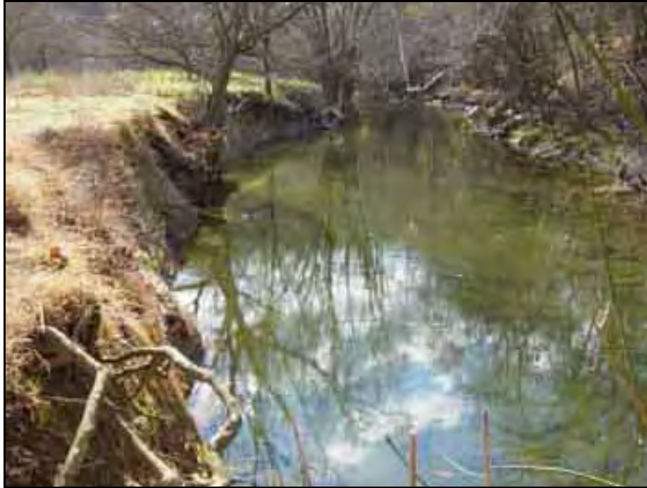
Erosion Location 3 (November 8, 2003)
