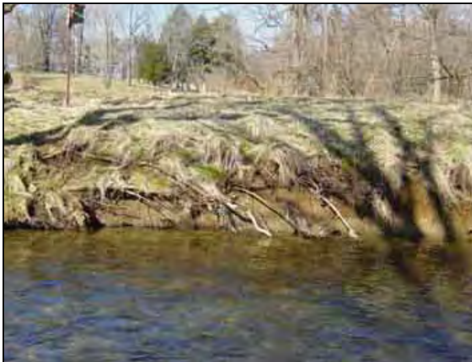
Erosion Location 24 (February 20, 2004)
