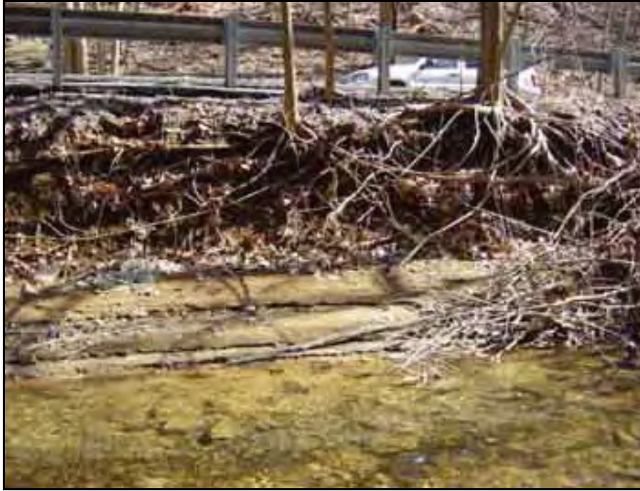
Erosion Location 19 (December 20, 2003)
