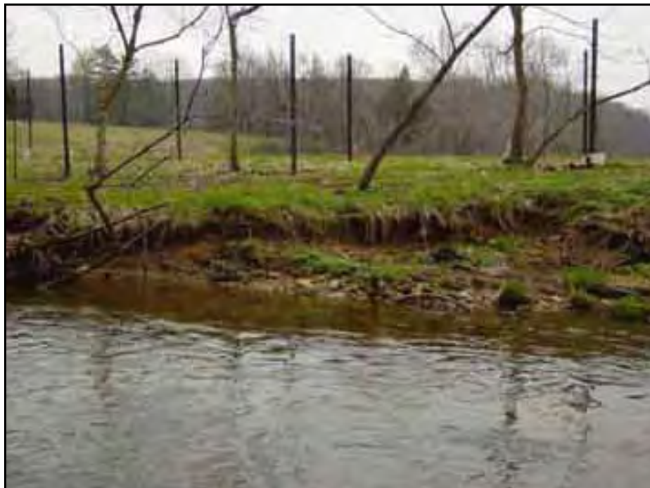
Erosion Location 30 (April 3, 2004)
