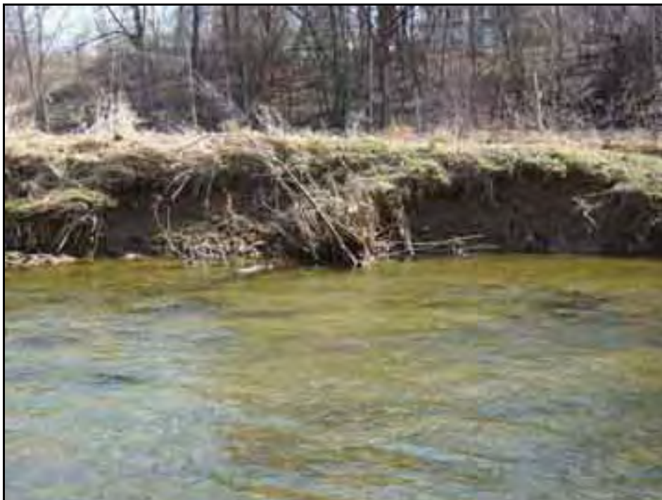
Erosion Location 26 (February 20, 2004)
