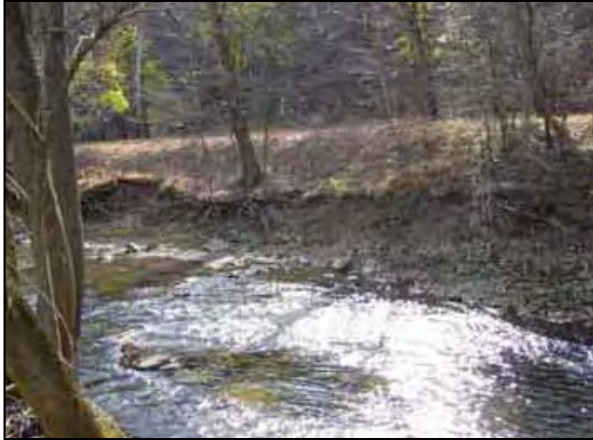
Erosion Location 5 (November 8, 2003)
