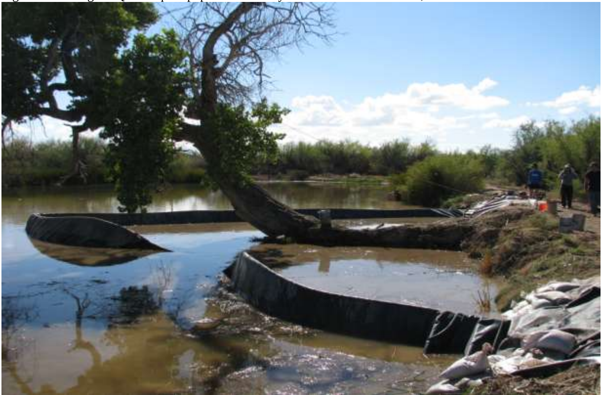
Figure 6. Cofferd dam failure. October 21, 2009.
