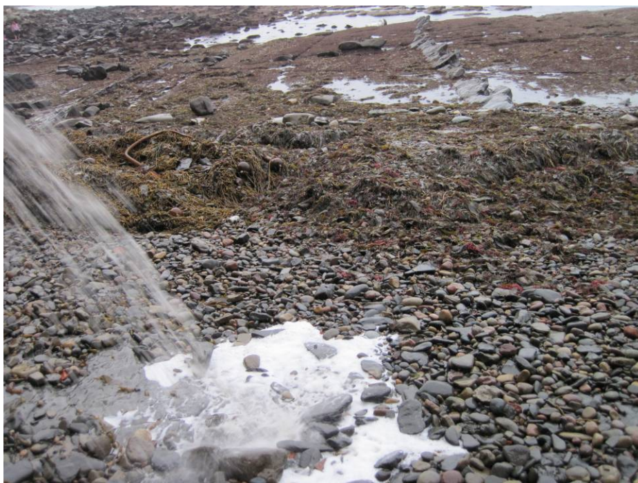
Figure 4. Flow of storm runoff during wet weather from storm drain pipe 186 at La Jolla Shores.
