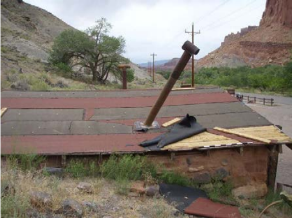
Merin Smith Implement Shed following Wind Damage
