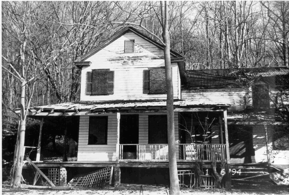
Pennyfield House c. 1994. Substantial damage had occurred by this time. (NPS/NCR)
