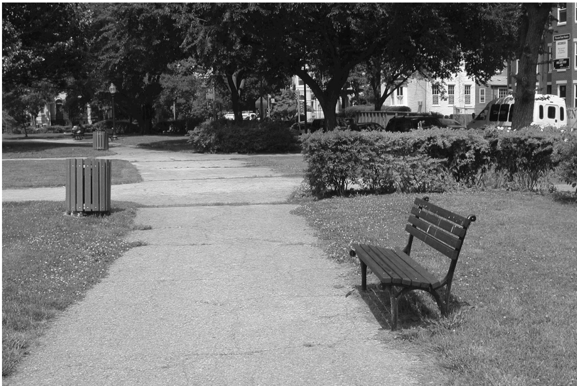
The 1936 bituminous concrete paving, chosen for its resiliency and dark, non-glare surface, still exists, though cracked and otherwise deteriorated. June 2004. (CLP digital photo, walk and bench BW 250)
