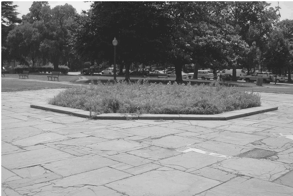
The fine workmanship and current poor condition of the plaza's fieldstone pavers are visible in this photo from June 2004. (CLP digital photo, plaza BW 250)
