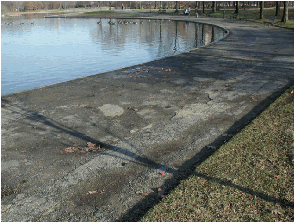
The walk circling the lake has lost much of its gravel, and the exposed asphalt is deteriorated. (Jan. 2007; CLP file)
