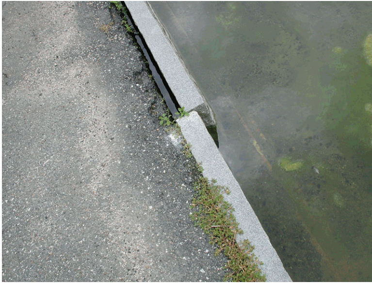
The granite walls that line the lake and create a curb along the lakeside walk occasionally pop from their anchors. This image also shows the heavy growth of algae that had developed on the water's surface by mid-June 2007. (CLP file)
