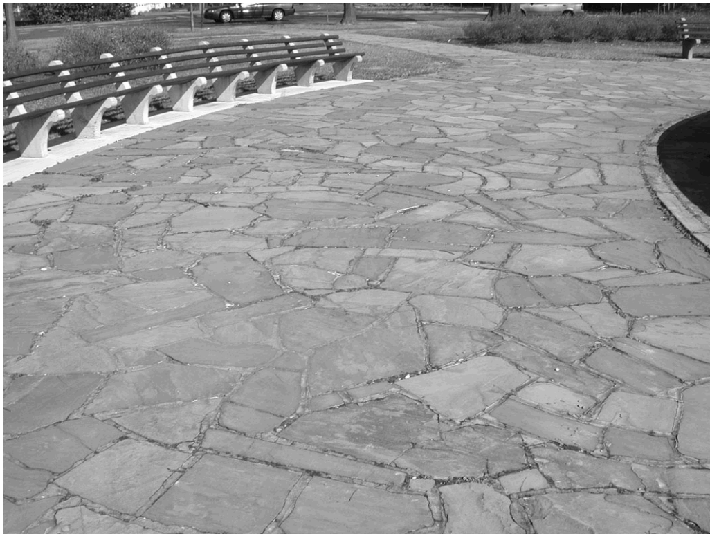
The deteriorated fountain plaza before the flagstones were reset/replaced. (CLP digital photofile, March 2002).
