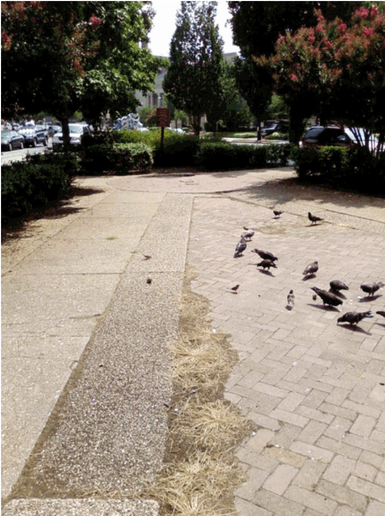
The brick internal triangle has settled beneath the internal walks, and soil and moisture is accumulating, causing weed growth. A visitor feeds pigeons here daily. (NCR CLP 2007).
