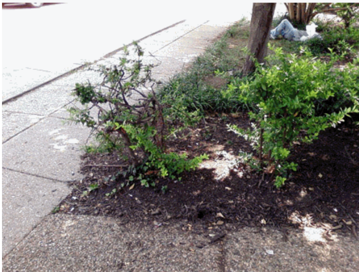
Heavy visitation and the resulting soil compaction has lead to thinning vegetation such as the pyracantha hedges (top and bottom) and holly trees (top). (NCR CLP 2007).
