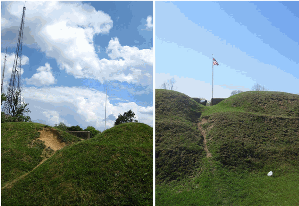
Erosion on the north side of the parapet (left: CLP June 2010; right: CLP April 2010).
