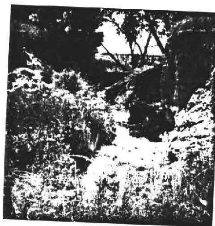
Thistle Dam 7-22-86 breeched dike (2)
