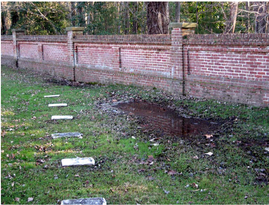
Figure 18. View of the inclosure wall at the south side of the cemetery where a low area creates drainage issues (SUNY ESF, 2006).
