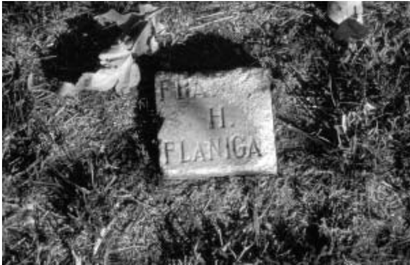
Figure 71. Cemetery marker in need of restoration, 2001.
