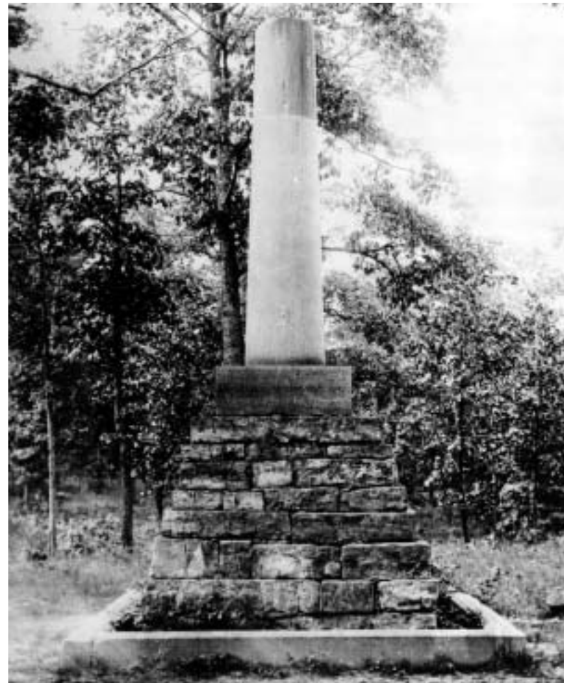
Figure 70. Meriwether Lewis Monument, c. 1916, showing invasion of weeds.
