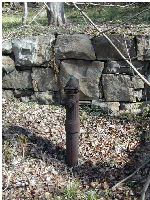
Water hydrant near the Nuttallburg church foundation ruins (OCLP 2003).
