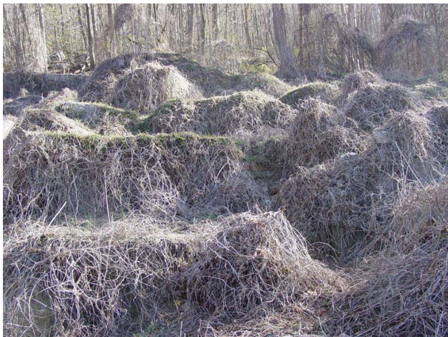
Kudzu blanketing retaining walls in the vicinity of the Clubhouse (OCLP 2003).
