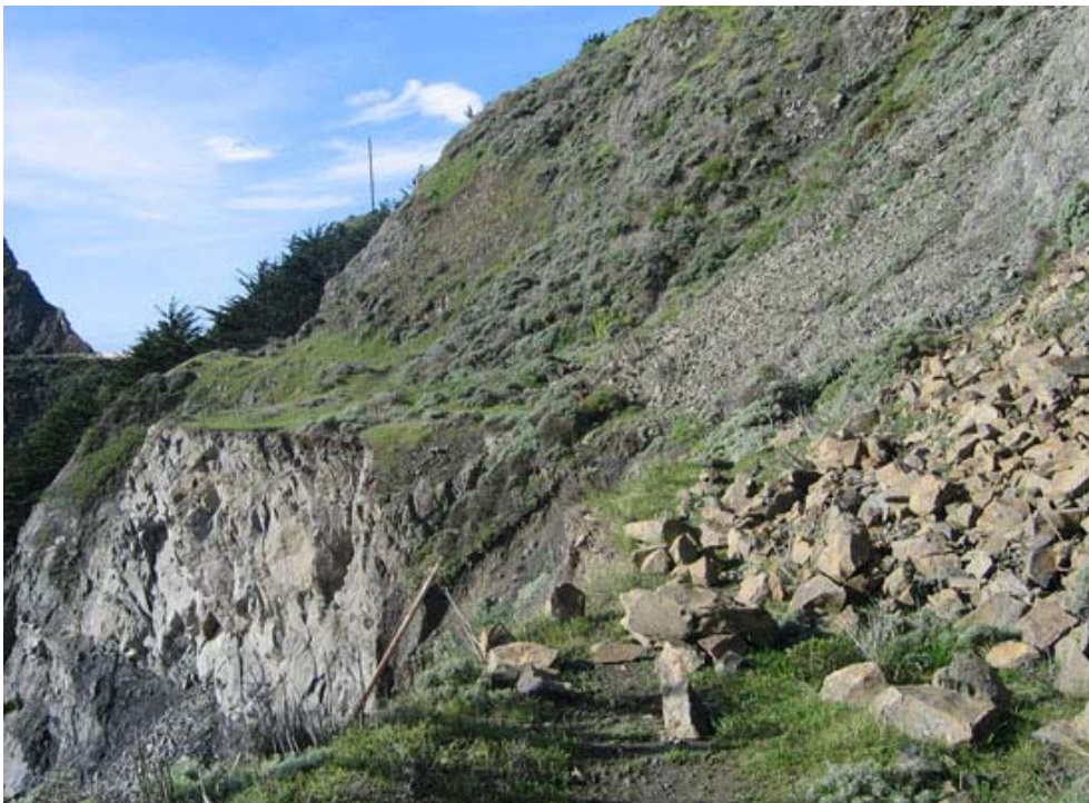
Circulation #2: View of one area of landslide damage found along the Boathouse Trail. (PWR, CLI, GOGA-D-2-22 047, 2005)
