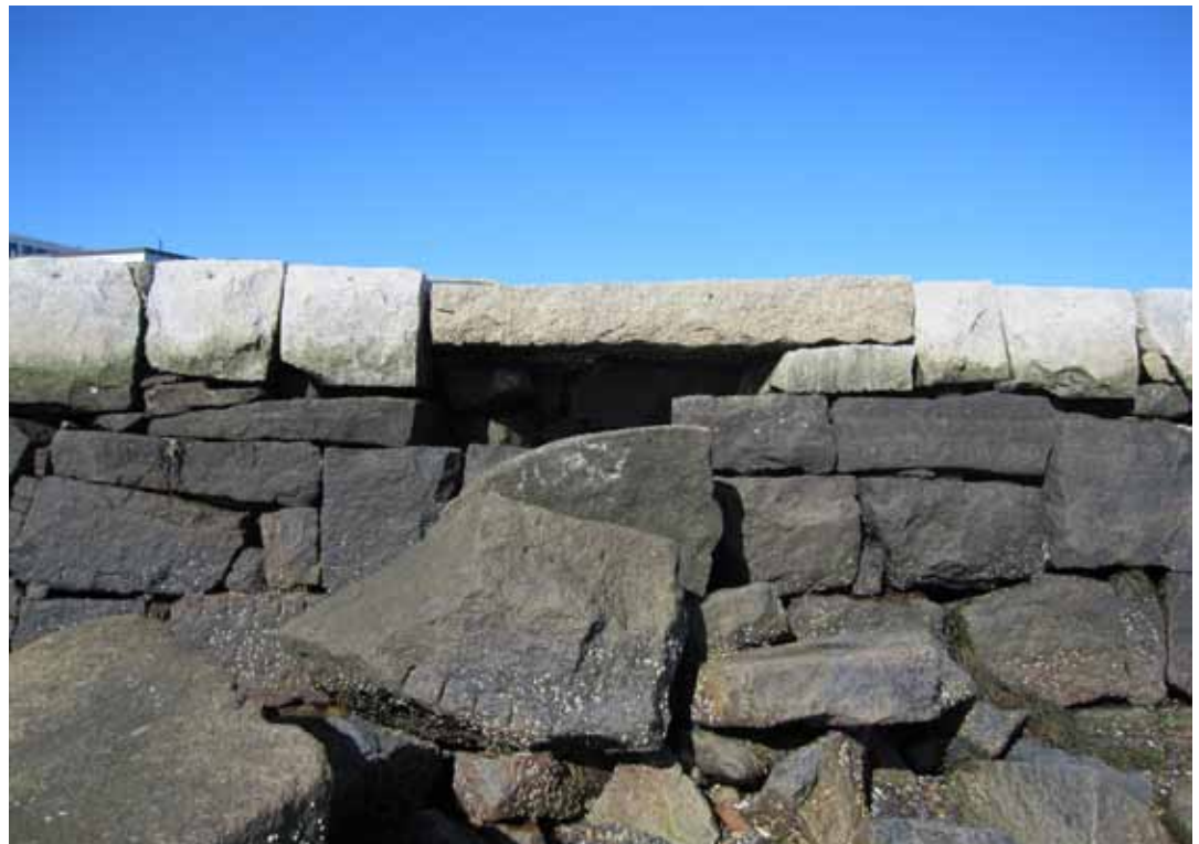
Sinkholes and other damage to Derby Wharf is a concern.
