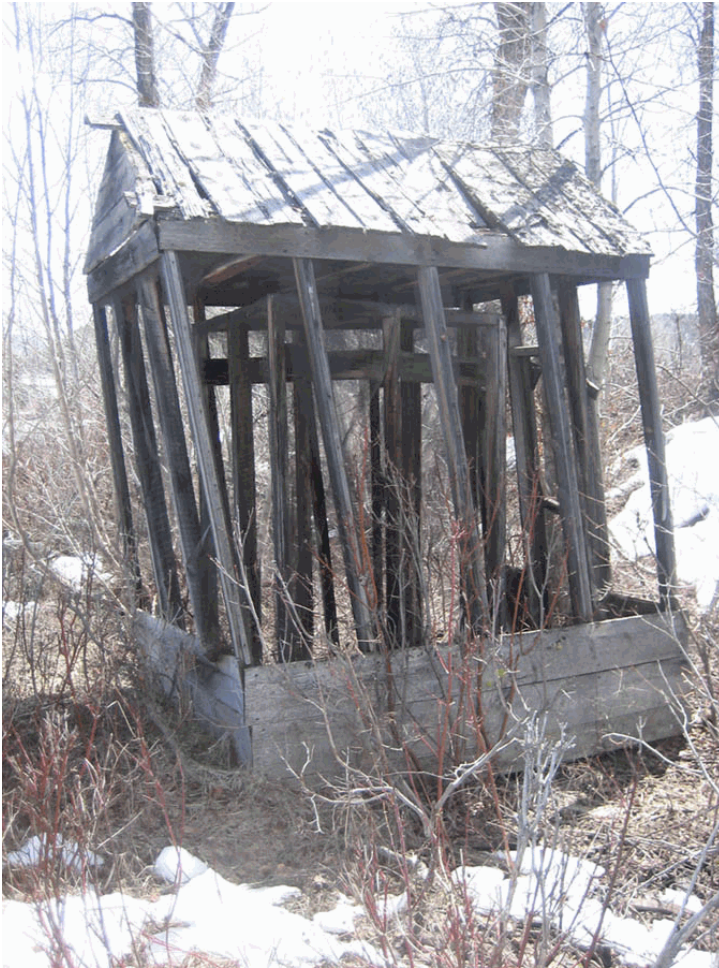
View looking east at curing house, 2010. Note significant deterioration of the structure. Source: C. Mardorf, NPS.
