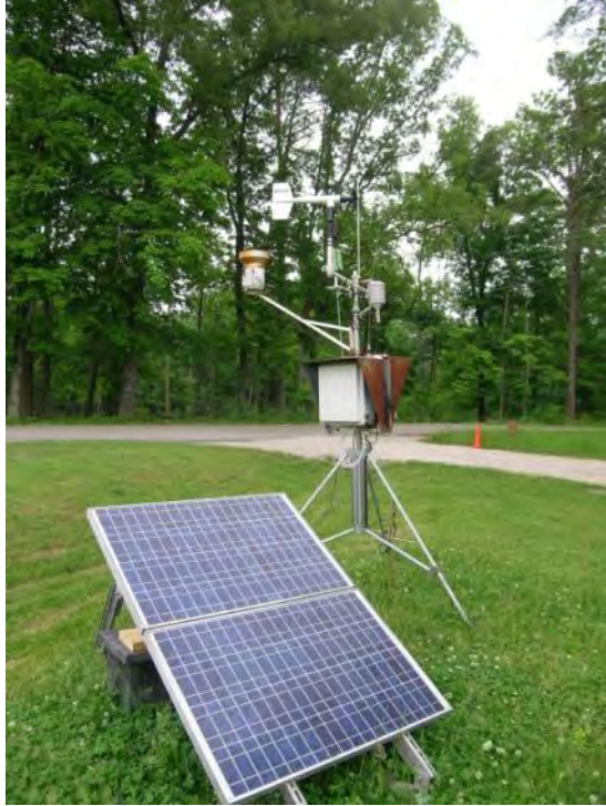
Figure 12. POMS II near CUPN's MACA office being prepared for its 2010 deployment at STRI.
