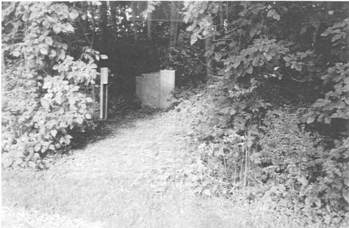
Figure 24: Electrical transformer, 1996 (OCLP).
