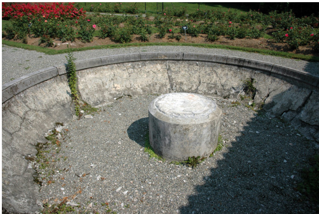
Figure 33. The shell of the Orpheus fountain in the lower rose garden is cracked and in need of repair (OCLP, June 2008).
