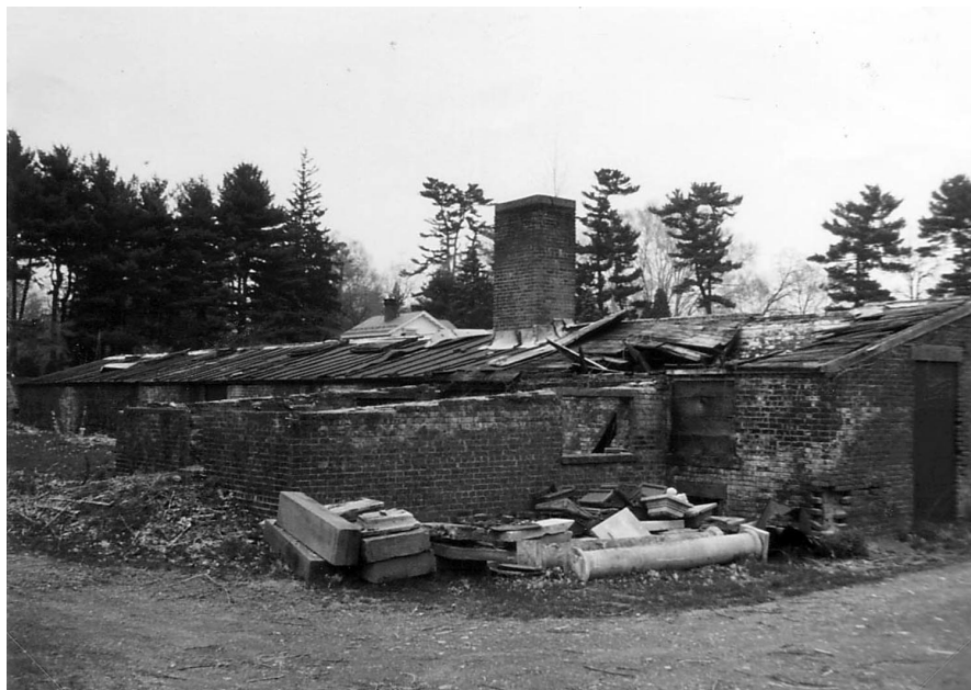
Figure 14. View looking northeast showing the damaged Potting Shed with stockpiled elements including columns and bluestone steps, circa 1970s (VAMA, no. 71592).
