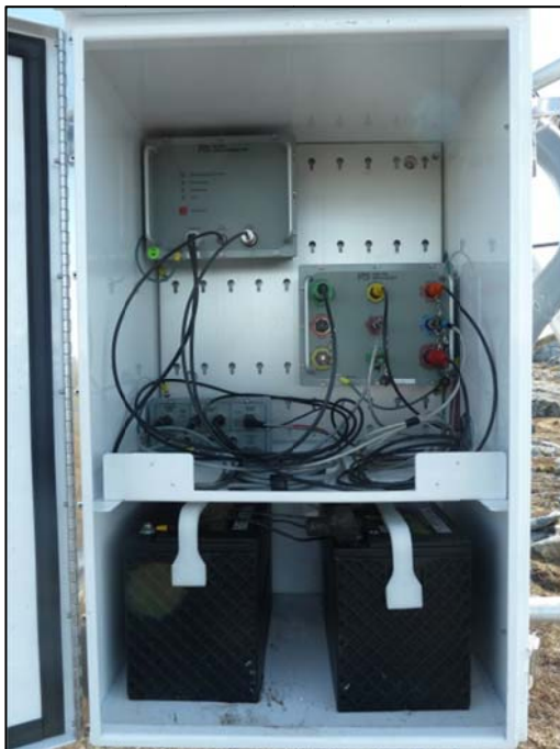
Figure 31. McArthur Pass RAWs - Inside of instrument enclosure photographed just before departure.
