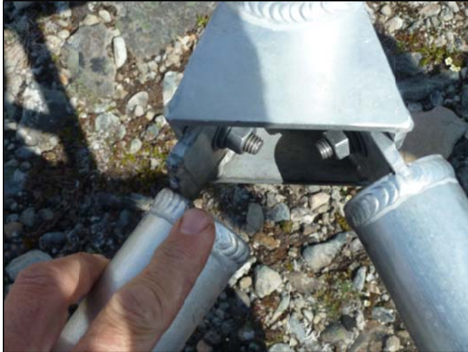
Figure 11. Fourpeaked RAWS – Broken weld on lower north corner of tri-leg tower frame.
