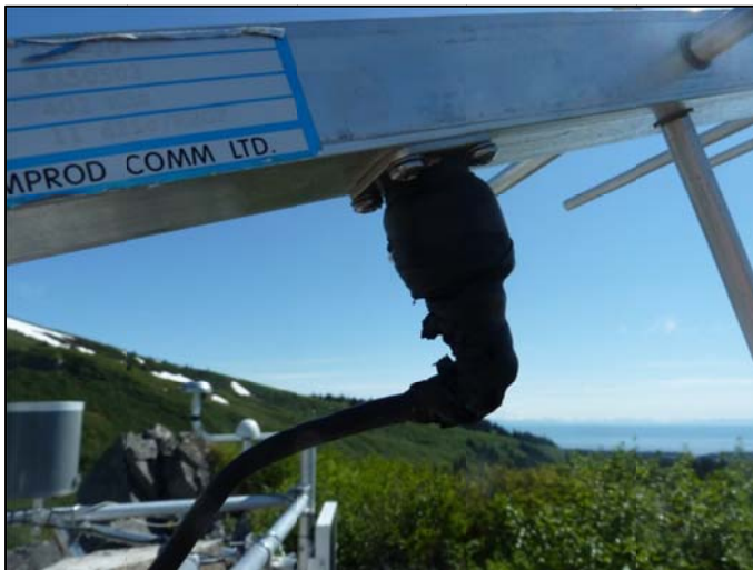
Figure 25. Hickerson Lake RAWS – The GOES antenna cable was chewed on.
