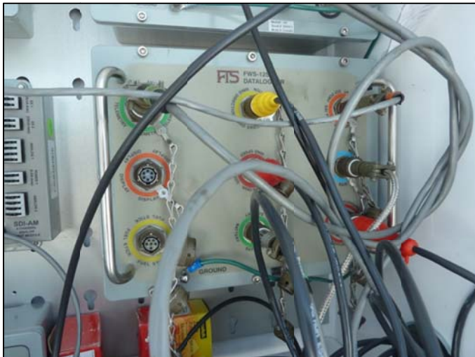
Figure 21. Harding Icefield RAWS – Inside of instrument enclosure photographed just before departure.
