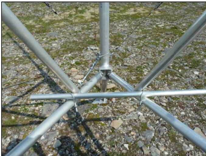
Figure 17. Fourpeaked RAWS – Aluminum pipe attached to help hold the broken tower frame welds together.
