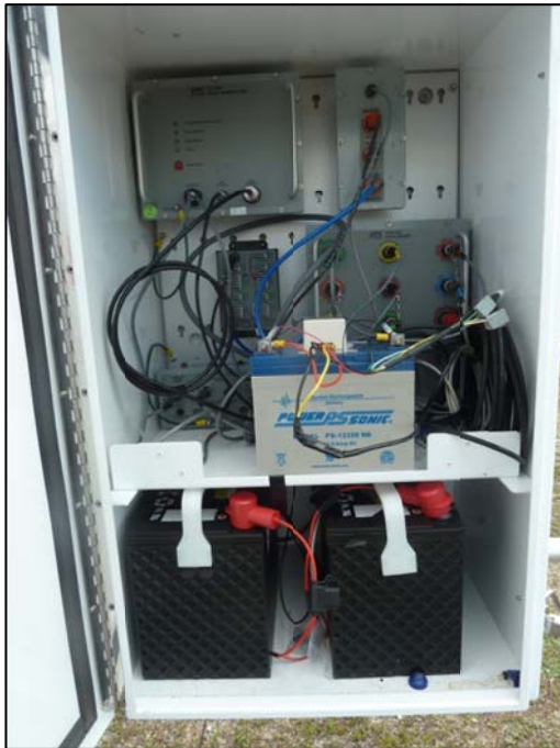
Figure 43. Snipe Lake RAWS – The inside of the instrument enclosure photographed just before departure. Additional 35 Ah battery for Campbell Scientific time-lapse camera is visible in the center of the photograph.
