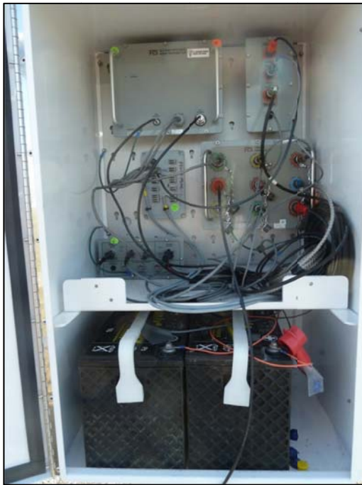
Figure 41. Pfaff Mine RAWS – Inside of instrument enclosure photographed just before departure.
