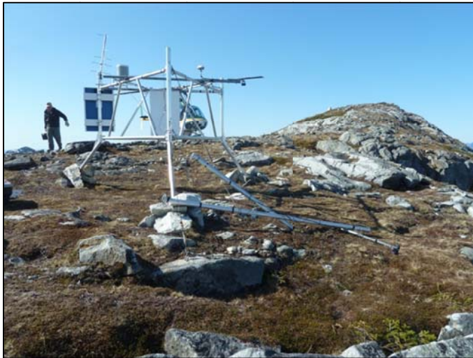
Figure 29. McArthur Pass RAWS – Broken 20-ft wind sensor mast.
