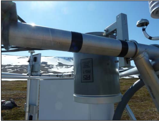
Figure 36. Pfaff Mine RAWS – The rain gauge tipping bucket was upside down and wasn't recording precipitation.
