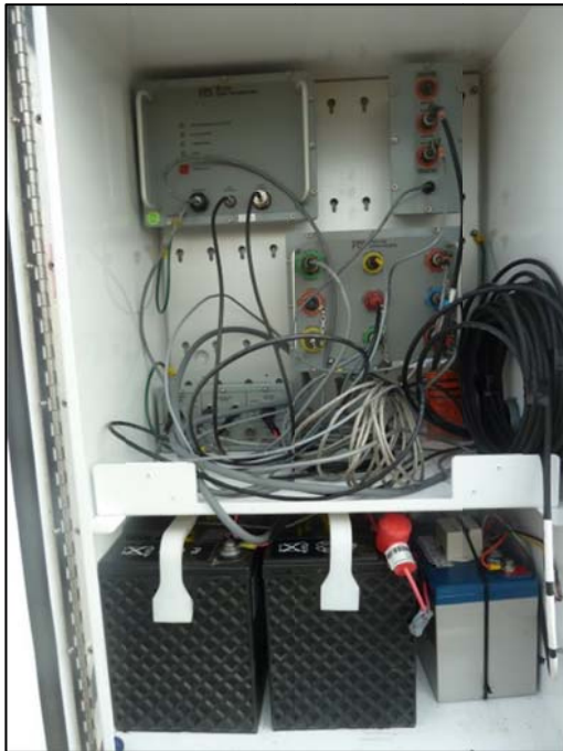
Figure 9. Coville RAWS - The inside of the instrument enclosure photographed just before departure. Additional 35 Ah battery for Campbell Scientific time-lapse camera is visible in the lower-right portion of the photograph.
