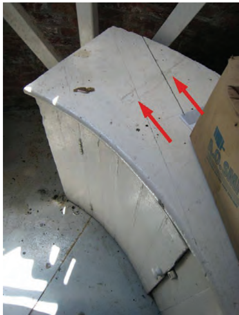
Figure C-93 Ghost marks of missing shelving supports.
