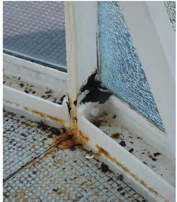
Figure C-98 Deteriorated iron framing.
