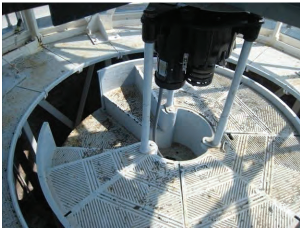
Figure C-97 Center cast-iron platform for beacon.
