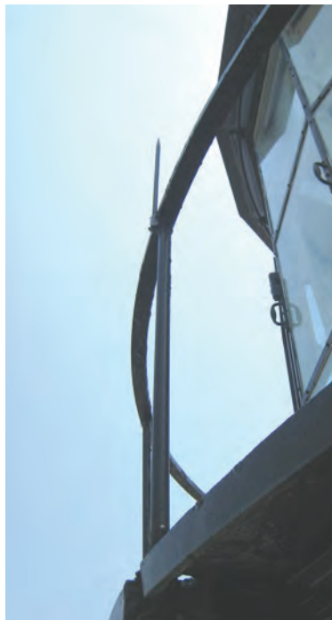
Figure C-36 Modern lightning rod at Gallery railing.
