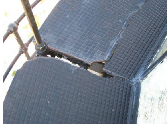
Figure C-23 Broken floor plates of Lantern Gallery.
