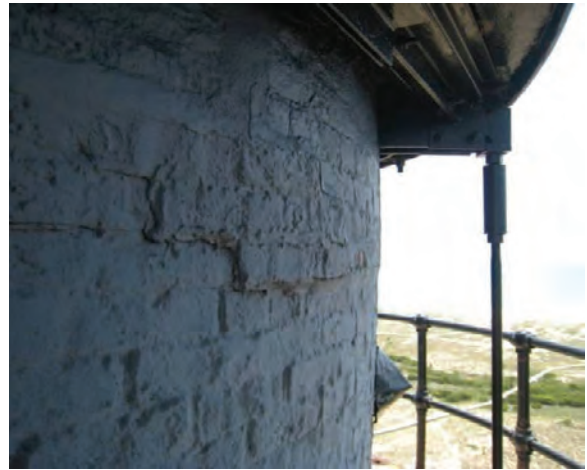
Figure C-107 Displaced masonry and supplemental tie rods.
