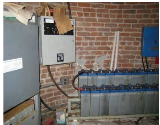
Figure C-58 Abandoned power controller and fuel cells.
