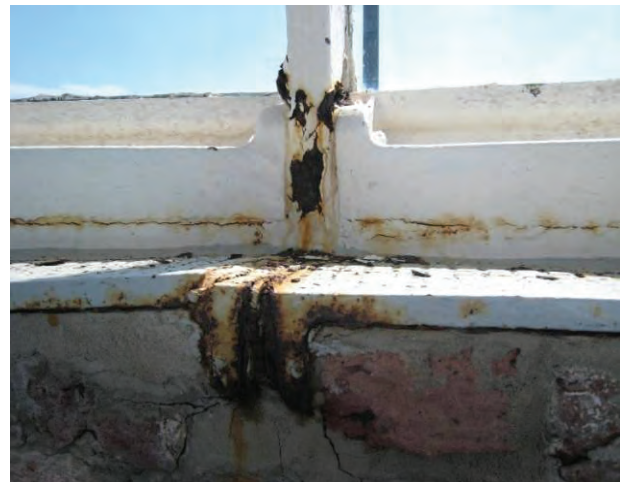
Figure C-104 Extensive corrosion of cast-iron framing.
