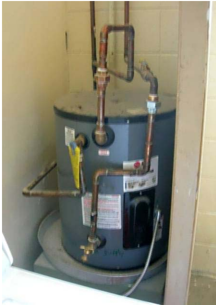
Figure 43: Unbraced Water Heater
