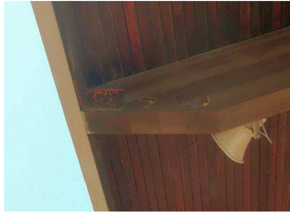
Figure 10: Rusted Hardware at Eave
