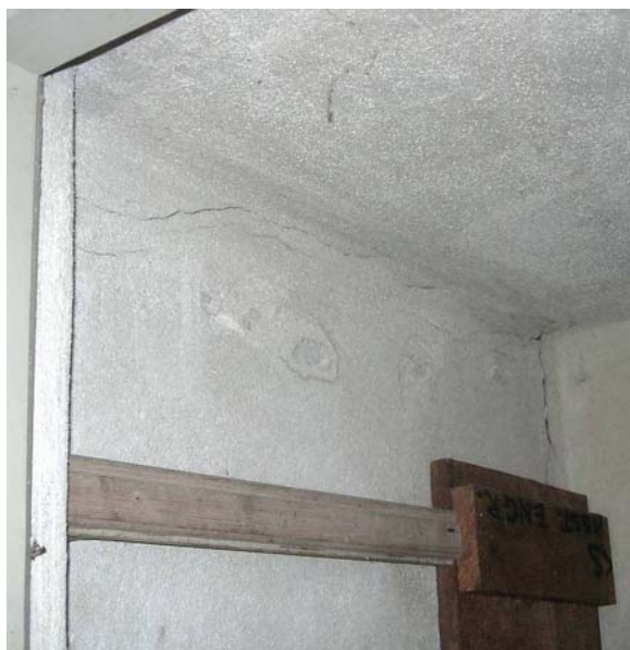
Figure 26: Crack at top of Basement Wall
