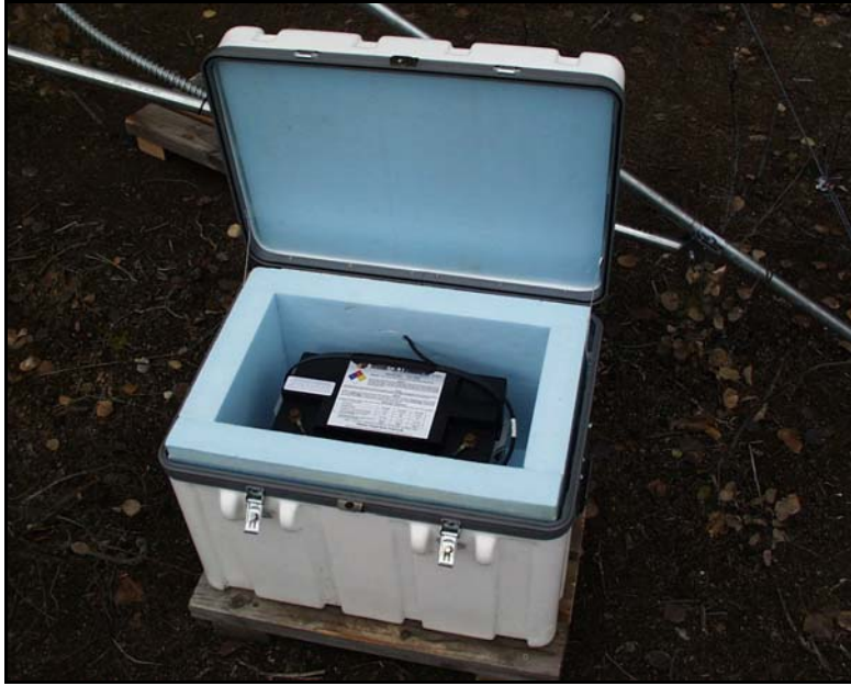
Figure 11. Battery and enclosure for CAKN station
