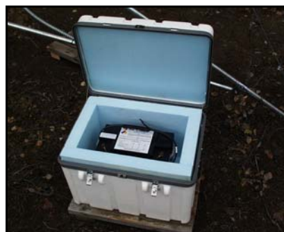
Figure 3 Battery and enclosure for climate station
