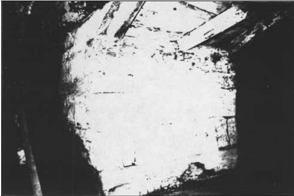
7. Room 001 Cribbed timber chimney footing
